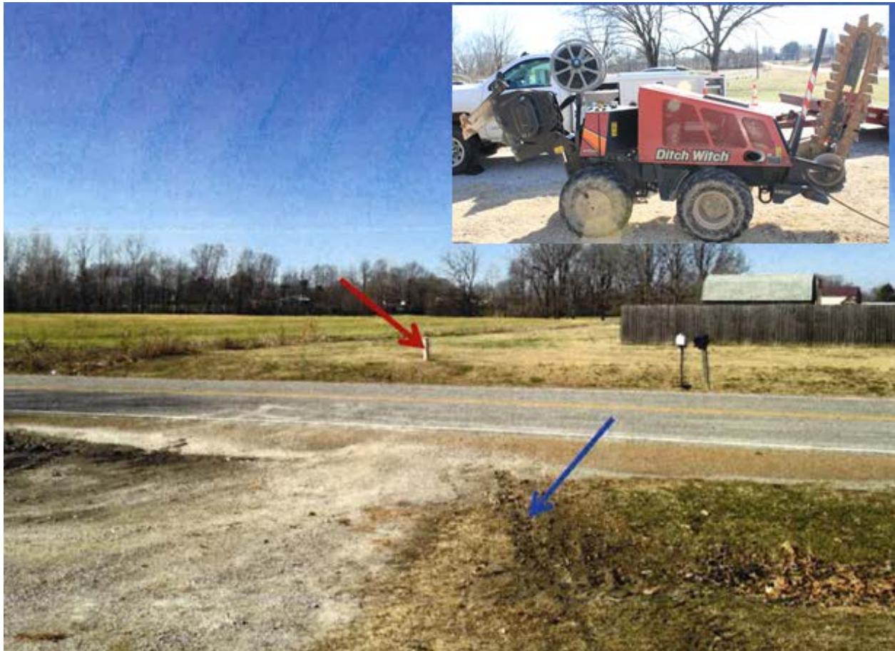
Photo 1 of 1 – View of the pedestal across the road, indicated by red arrow, and the approach trench filled in with dirt, indicated by blue arrow. View of the ditch witch used to dig the trench.
