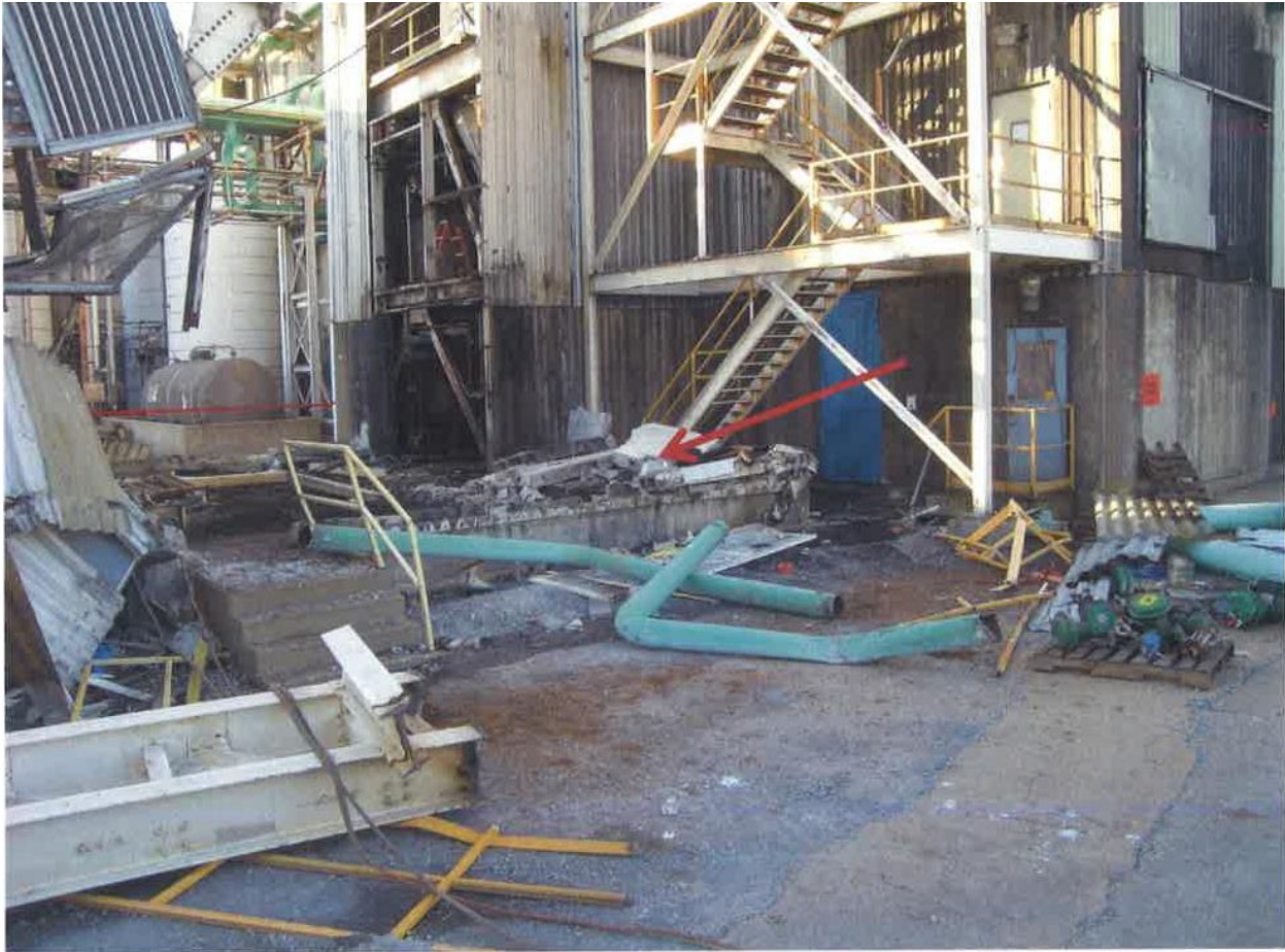
Photo 1 of 1: Southeast side of the Fructose Building after the Carbon Column Area collapsed. The cement masonry wall that struck the victim is designated by the red arrow.
