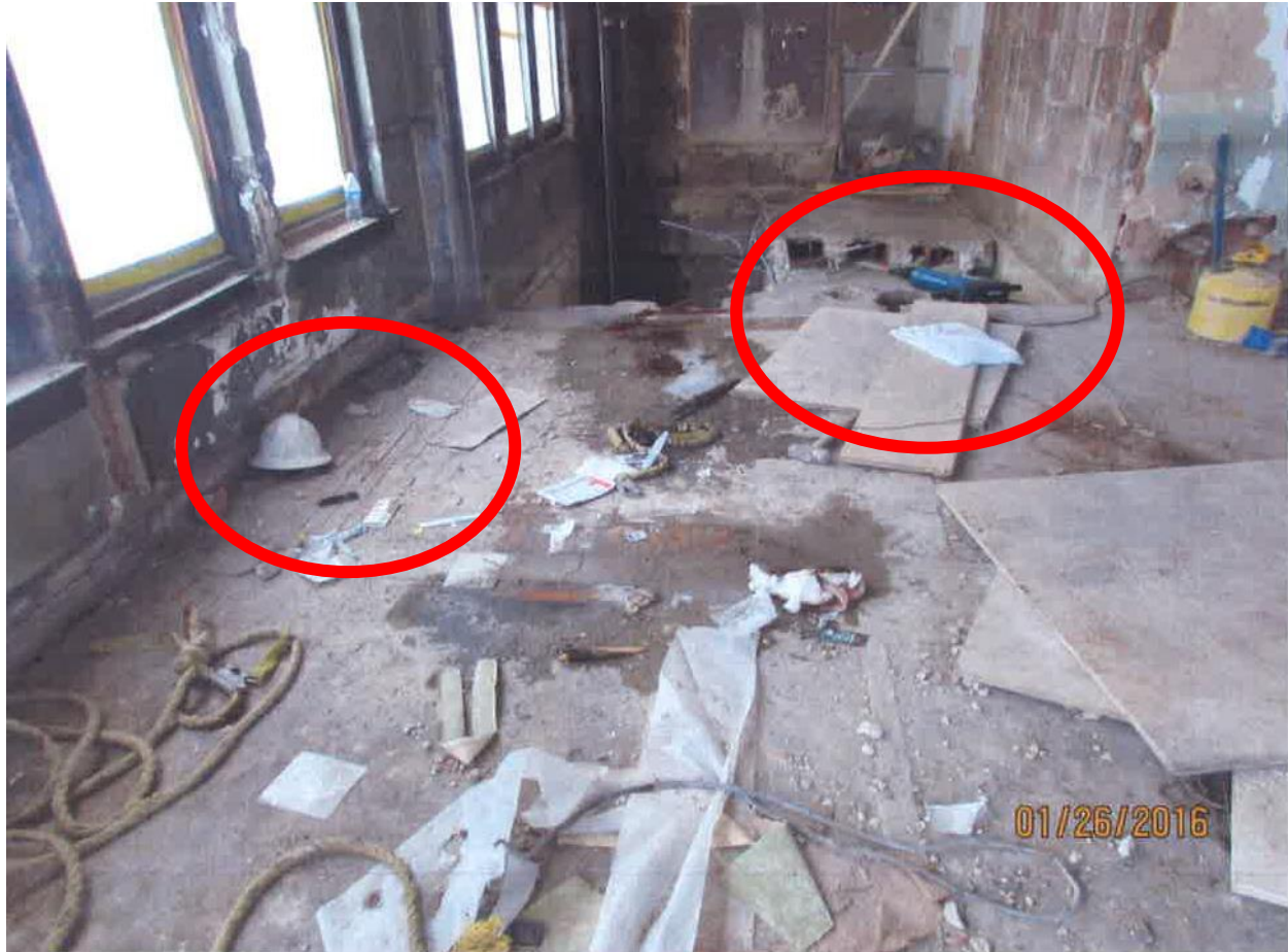
Photo 1 of 1 – Photo shows the location of the jackhammer and hardhat
