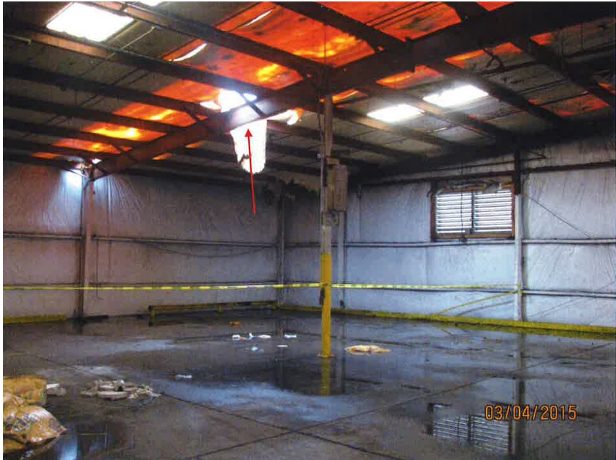
Photo 1 of 1 – Photograph showing the hole the victim fell through.
