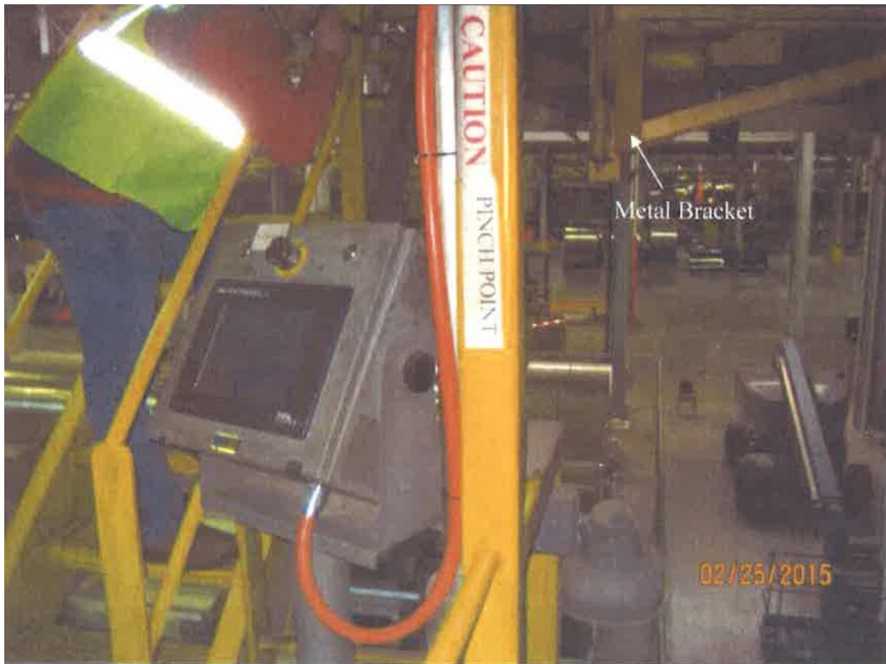
Photo 1 of 2 – This photo is a view of the platform where the open cab and panel are located for the crane.
