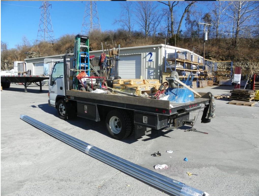
The victim was struck in the head by shifting fence rails while loading the work truck
