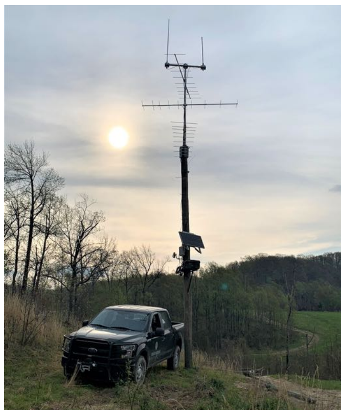
TWRA MOTUS tower at Massengale Mountain on North Cumberland WMA for monitoring migratory birds / David Hanni, TWRA
