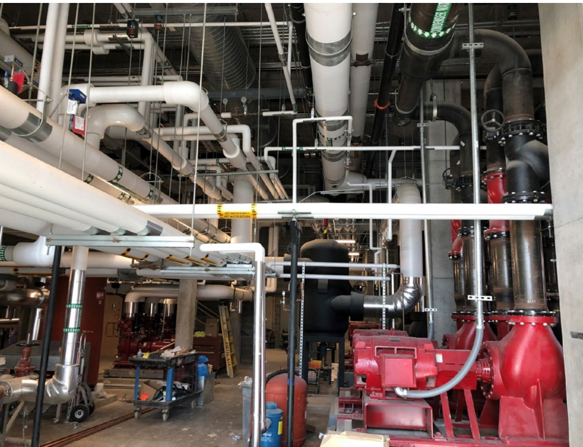
▲ Zeanah Chiller Plant
