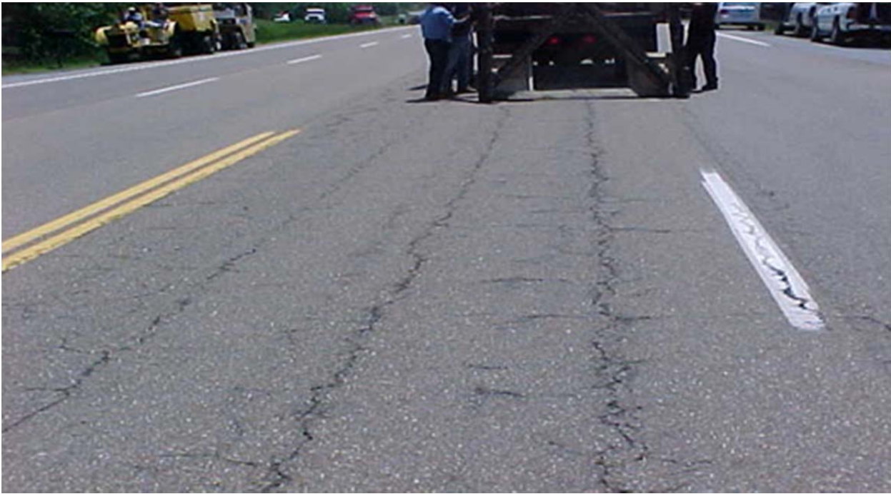
Extensive cracking from oxidation, no structural damage
