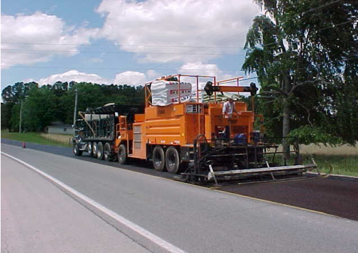
SR 290 - Putnam County – Minor rutting and cracking. Single course micro-surface.
