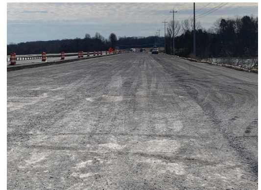
Section south of Academy Road is ready for asphalt paving when weather allows.
