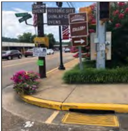
Figure 12: Sidewalks in need of repair
