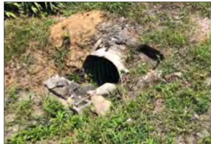
Figure 14: Inadequate Stormwater Infrastructure
