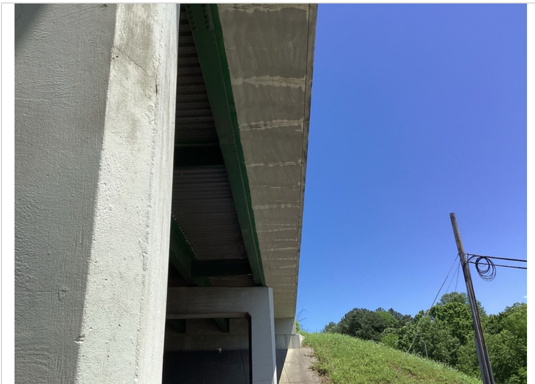
All spans transverse cracks with efflorescence right overhang
