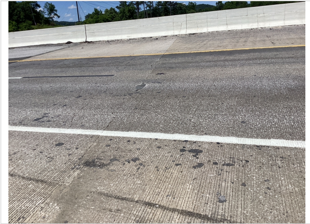
R A approach cracking on deck
