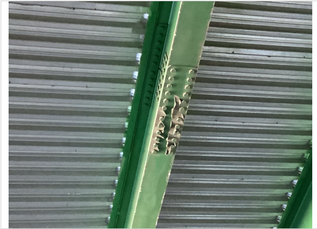
Span 2 beam H at splice plate-flaking paint
