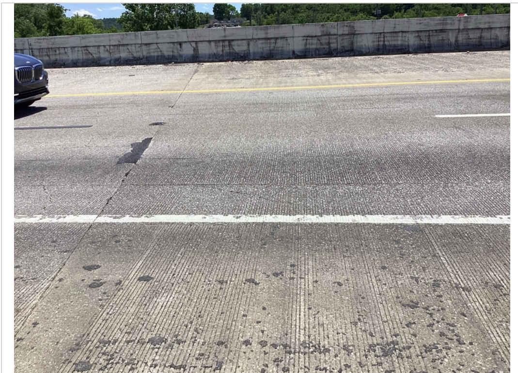
L B approach crack on deck
