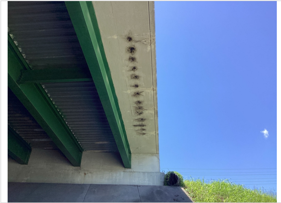
Span 1 left overhang near abutment some minor spalls with exposed steel
