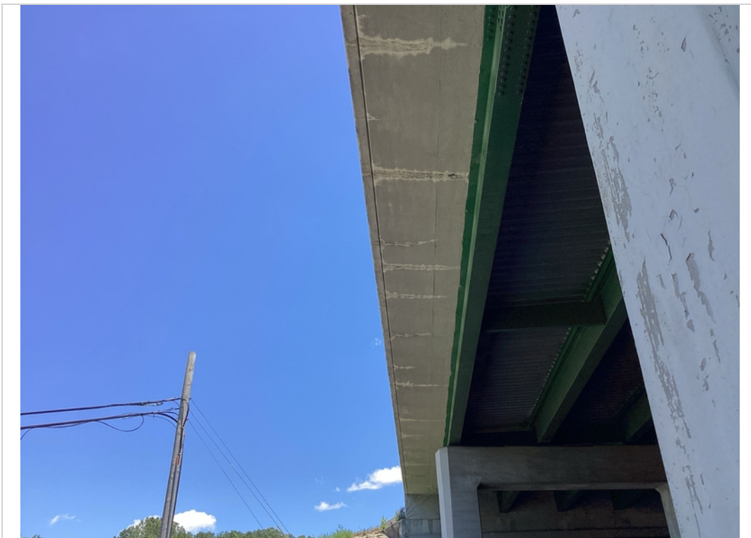
All spans transverse cracks with efflorescence left overhang
