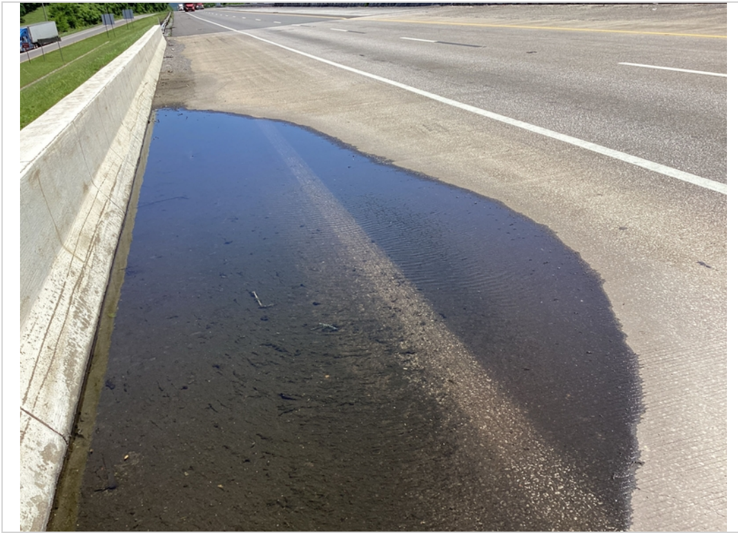
L A approach left side pooling water on deck
