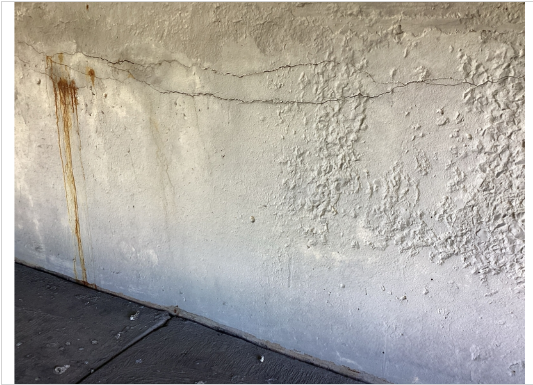
Abutment 1 LT horizontal cracks w/ rust staining
