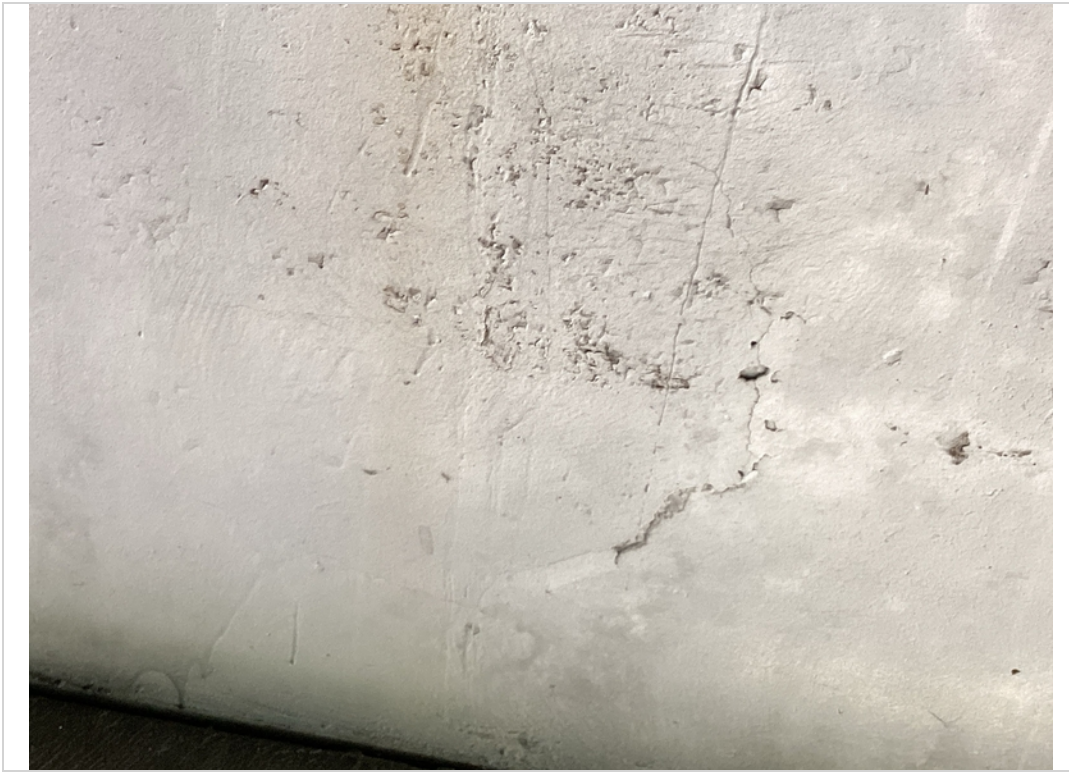
Abutment 1 cap area of Delam under beam F
