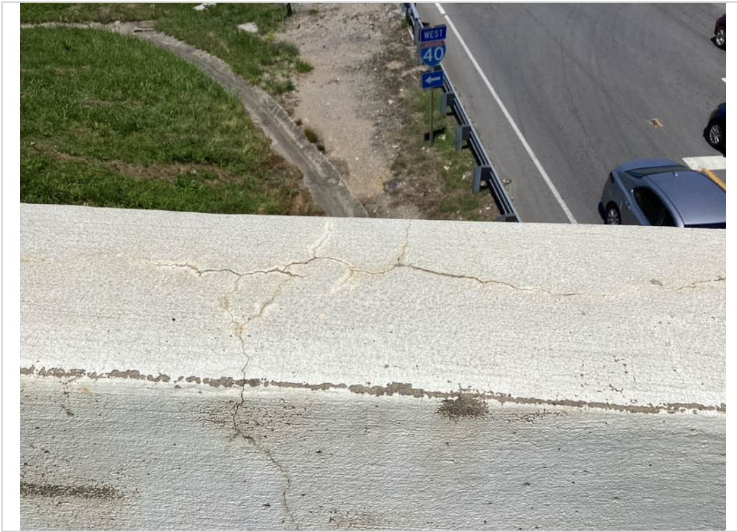
L Span 1 left side map cracking
