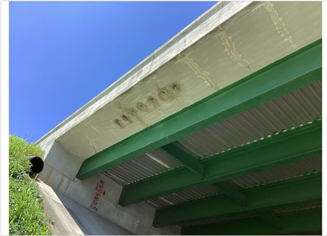
Span 1 right overhang near abutment some minor spalls with exposed steel
