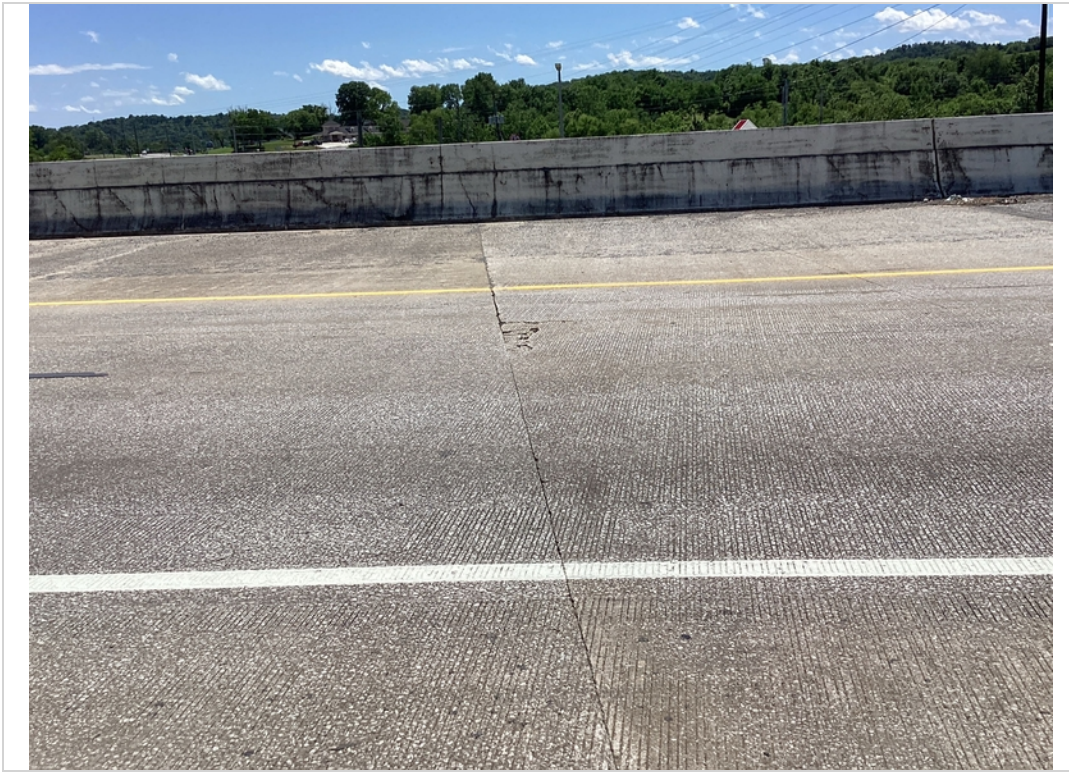
L A approach crack on deck
