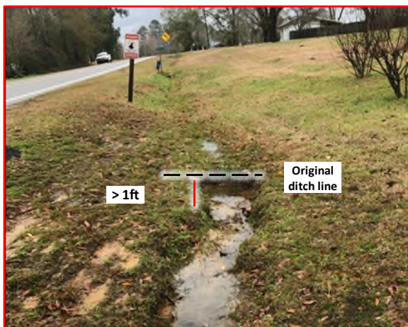
UNPAVED DITCH EROSION
