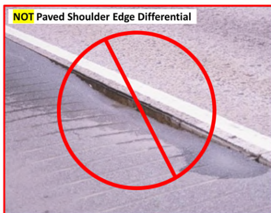
This is settlement. Note the “sinking” effect in the pavement.
