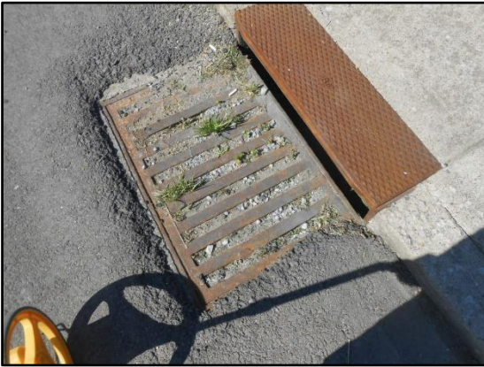
Example: An inlet fully obstructed.
