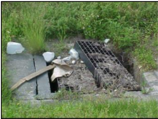
Example: Grate is out of the cradle.
