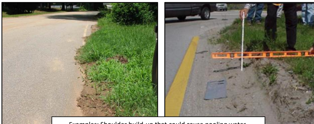
Examples: Shoulder build-up that could cause pooling water.
