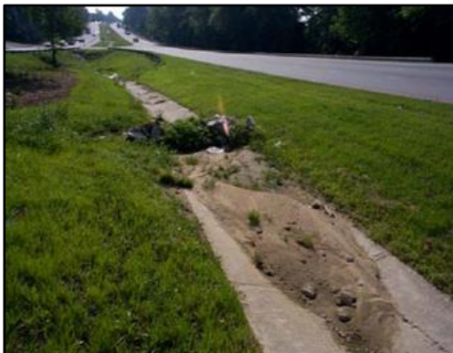
Example: Paved ditch with >50% of depth blocked by debris for 50 continuous feet.
