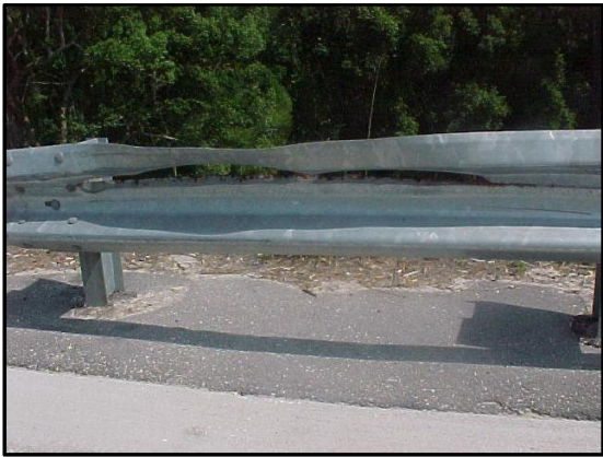
Example: Guardrail penetrated by a crash.
