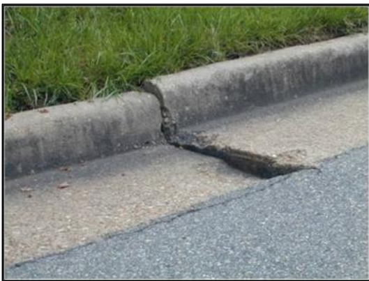
Misalignment greater than two inches does not meet the MQA threshold.
