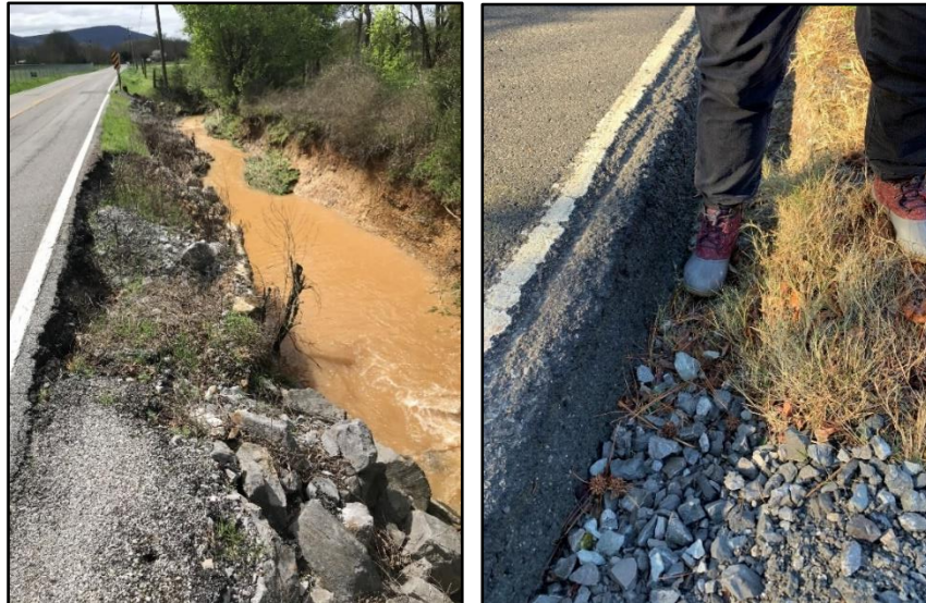
Examples: Any shoulder drop-off exceeding 4 inches.
