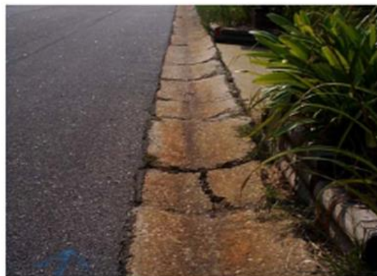
Example: Unsealed cracking greater than \frac{3}{4} inches.
