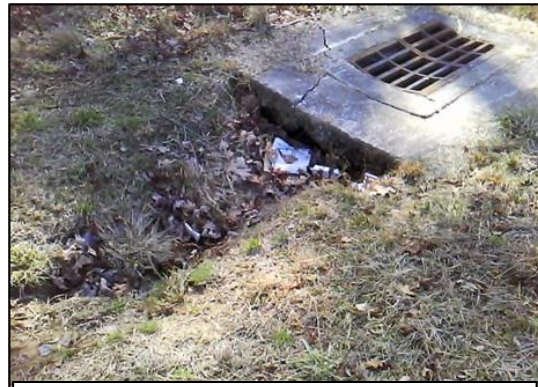
Example: Not a paved ditch, but example of undermining of a paved slab.
