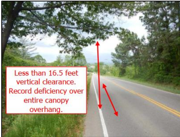
Example: Trees overhanging roadway and shoulder within 16.5 feet does not meet the desired condition.
