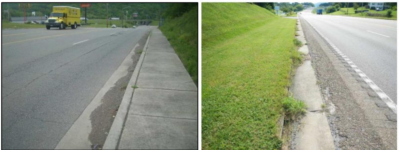
Example: Material accumulation in curb and gutter.
