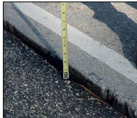
Paved Shoulder Drop-off – example of drop-off from rigid pavement travel lane to flexible paved shoulder
