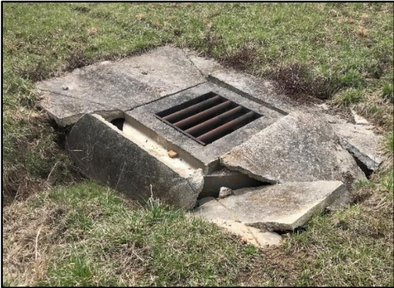
Example: Cracking and misalignment of concrete apron.
