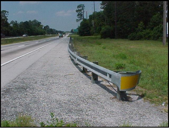
Example: Guardrail with damaged end section.
