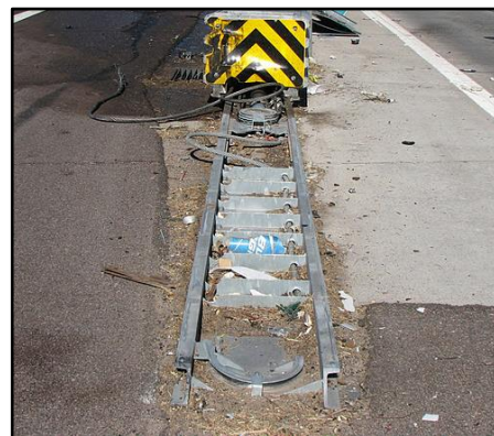
Example: Impact attenuator not operational. Source: AZDOT
