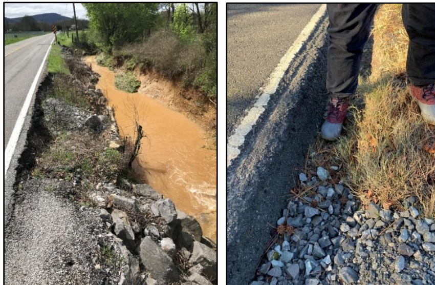
Examples: Any shoulder drop-off exceeding 4 inches.
