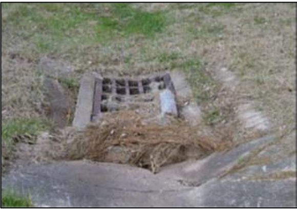
Example: More than 50% of the inlet is blocked.
