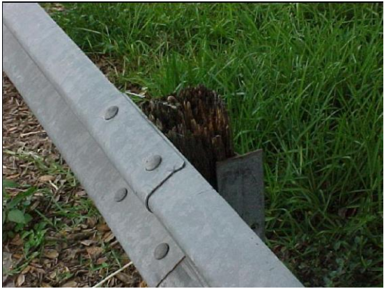
Example: Rotted offset block.
