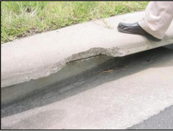
Example: Exposed steel in curb inlet and greater than 0.5 SF fails to meet the desired condition.
