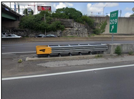
Example: Operational impact attenuator.
