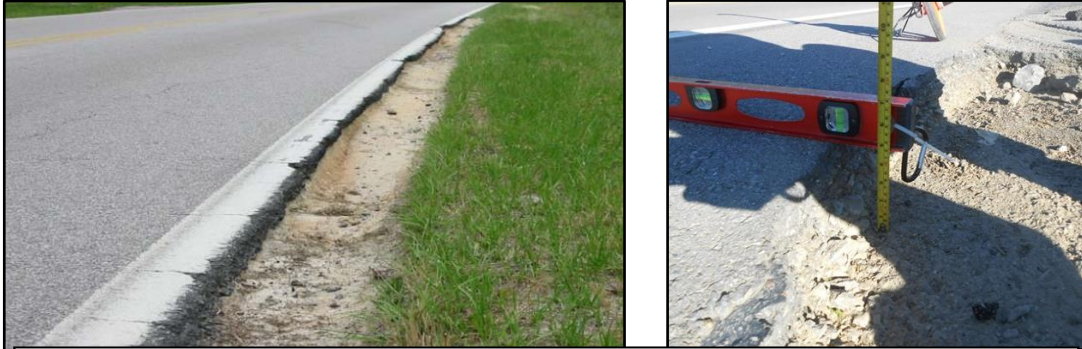
Examples: Shoulder drop-off exceeding 2 inches within 1 foot of pavement edge for 25 continuous feet.
