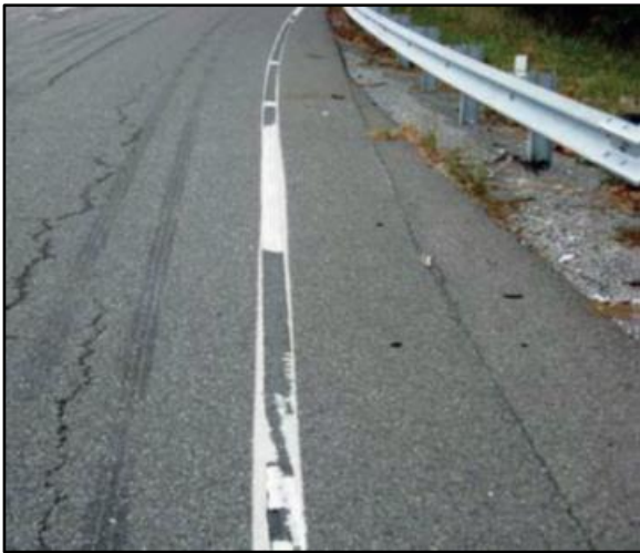
Example: More than 10% of striping has worn off.
