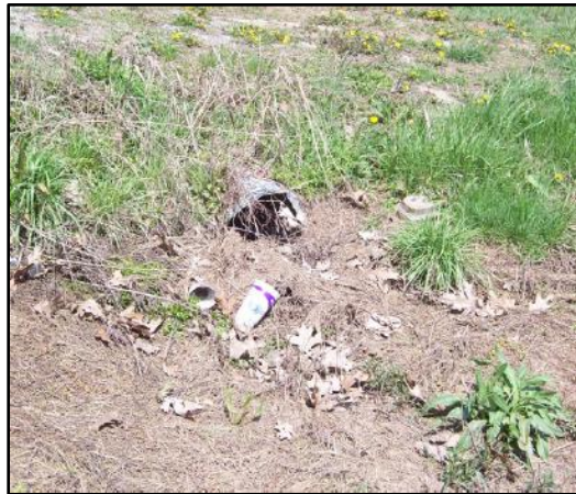
Material blocking this paved ditch is greater than 50% of the ditch depth.
