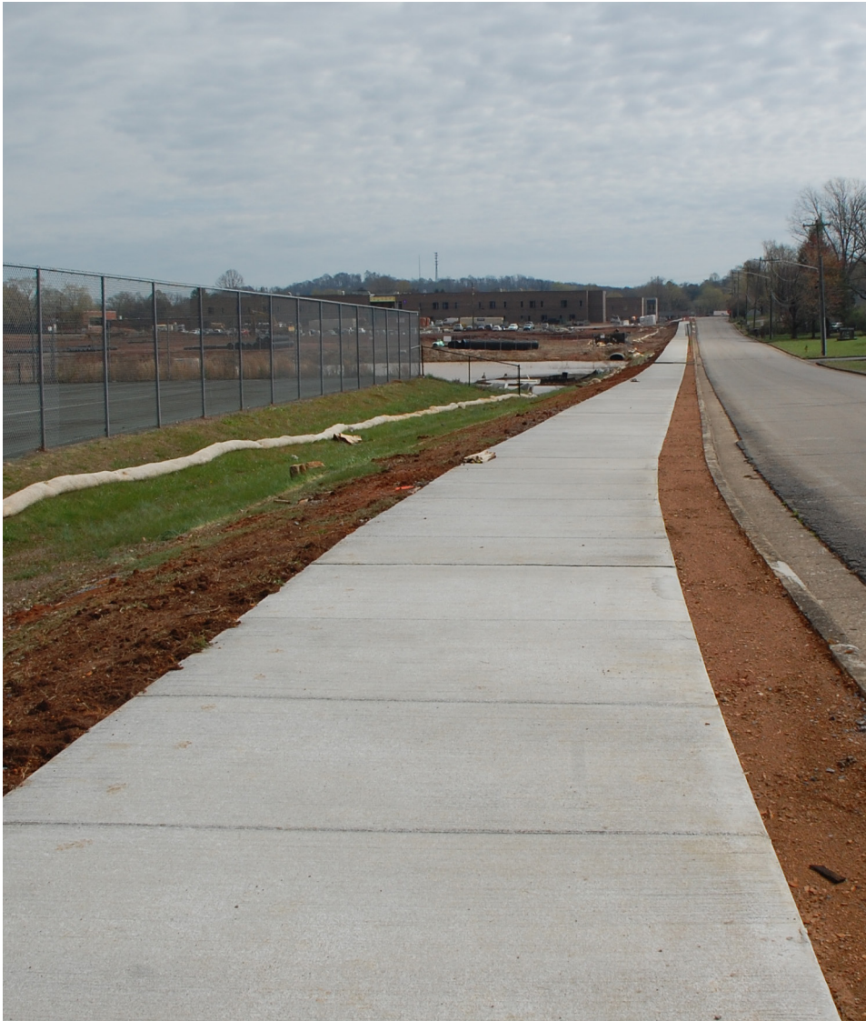
Shared-Use Path currently under construction at the Athens City Schools property. This path was recommended in the 2021 Community Mobility Plan.
