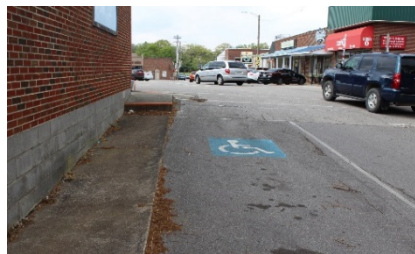
Figure 10: ADA Noncompliance Issue
