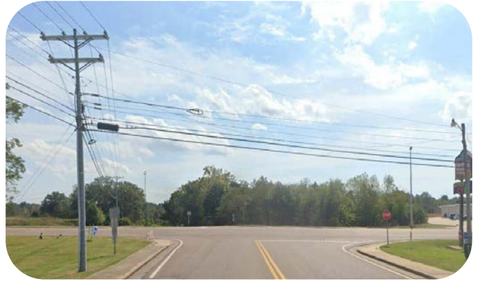
POWERLINES ALONG EAST SIDE OF LINDEN ST.
