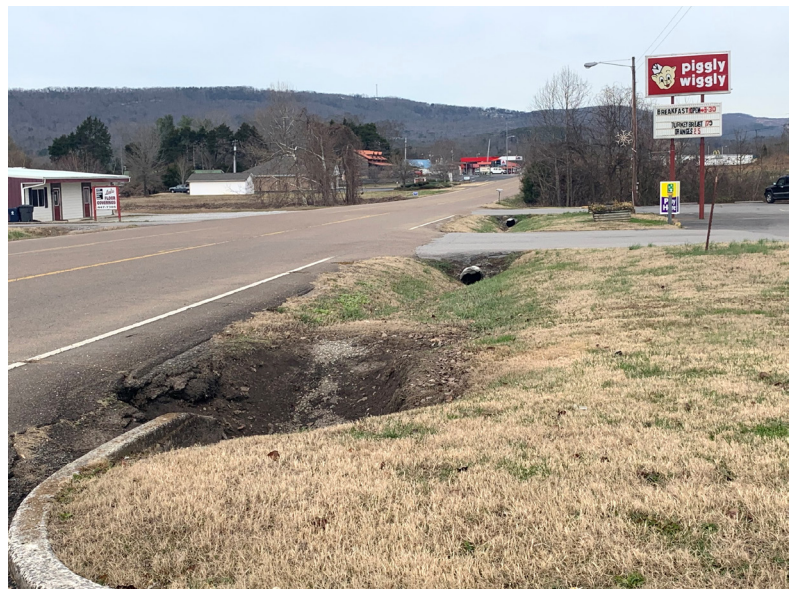
Roadside drainage would be improved through the addition of sidewalks, curb and gutter as outlined in Option 4.
