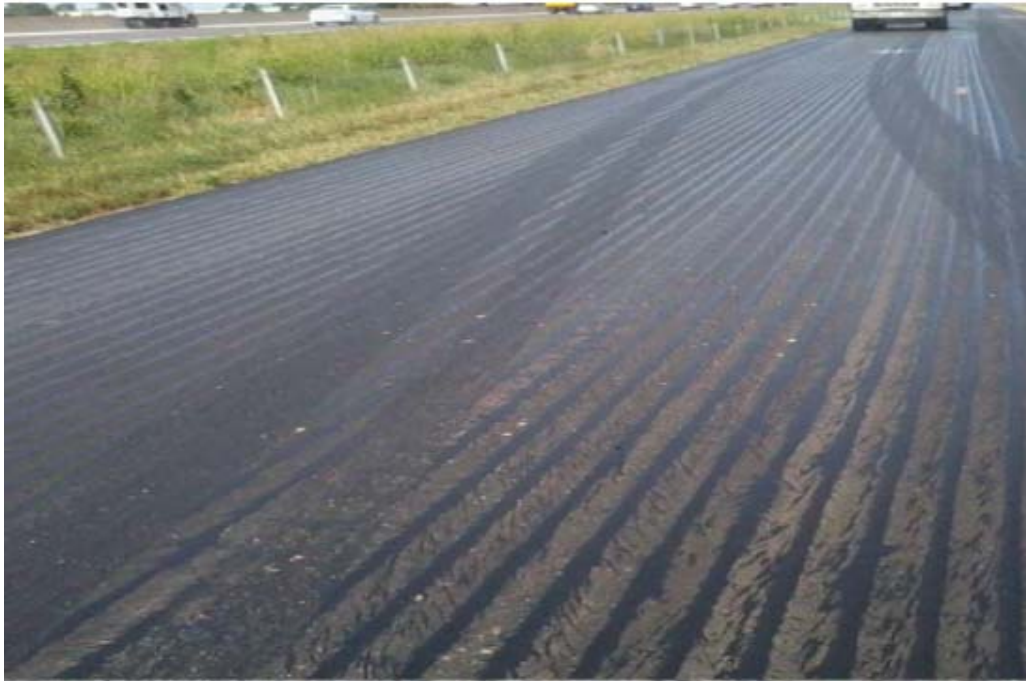
Improper Tack Coat, Zebra Strip/Corn Rows. Unacceptable.
