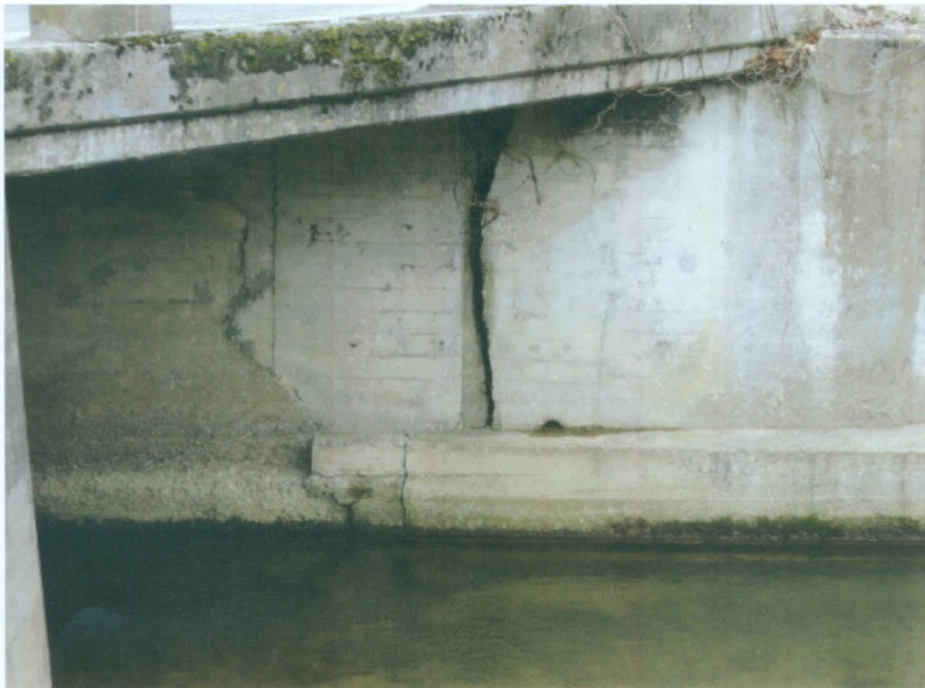
CRACKING IN THE ABUTMENT
