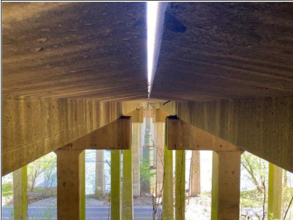
Gap between the two bridges
