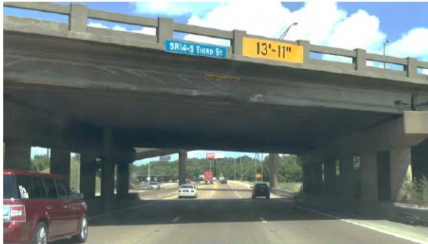
I-55 approach, looking eastbound, clearance 13'11", damage
