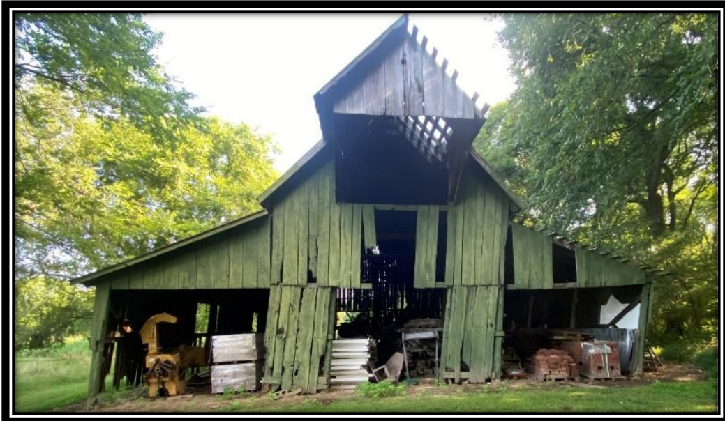
East Field Barn condition September 2025. Note lean of building to the east and missing metal roof panels and wood siding, September 2025.
