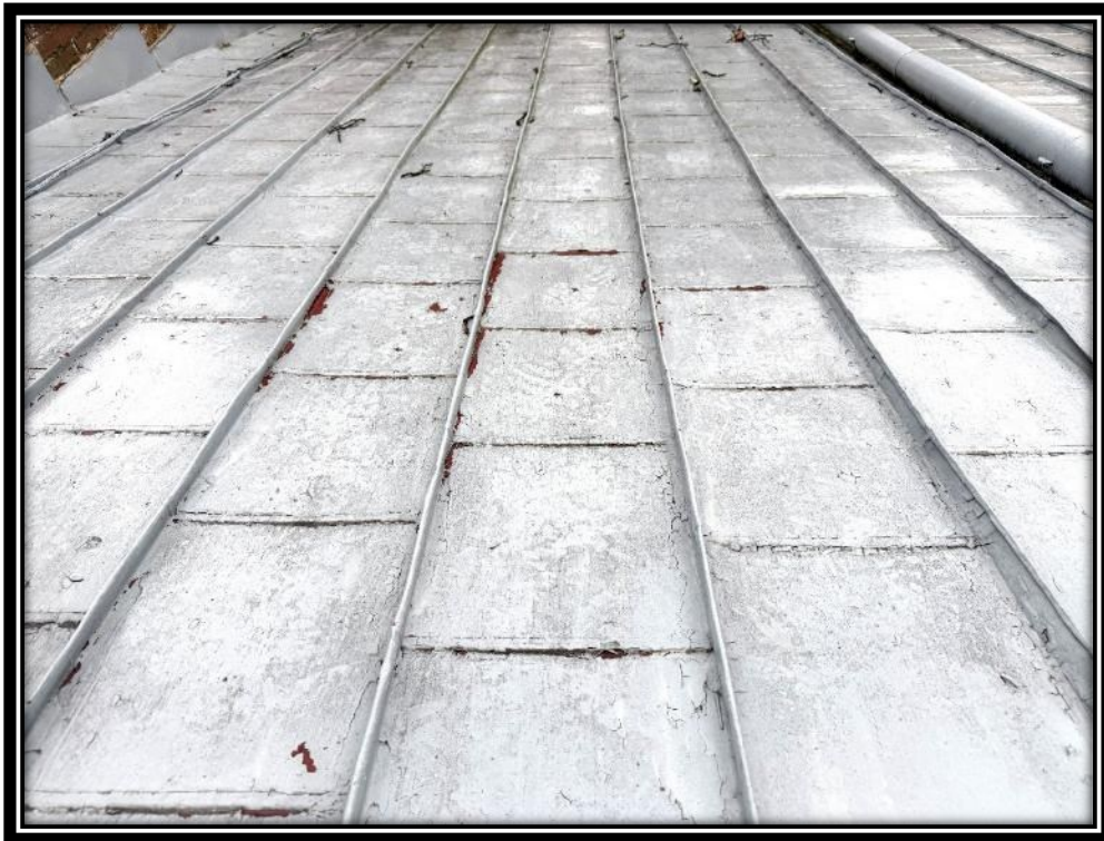
Roof paint on the Hermitage's west wing roof shows cracking and chipping, December 2025.
