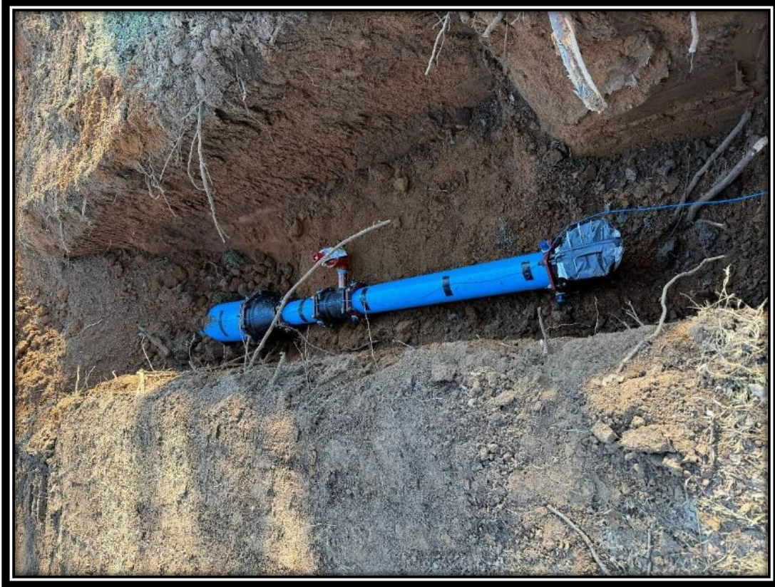
Reducing valve and backflow connection on the new water line at its end point at the Site Operations Facility, December 2025.
