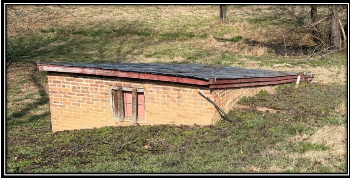
Pumphouse south and east elevations with site of former fire pond in background, December 2025.
