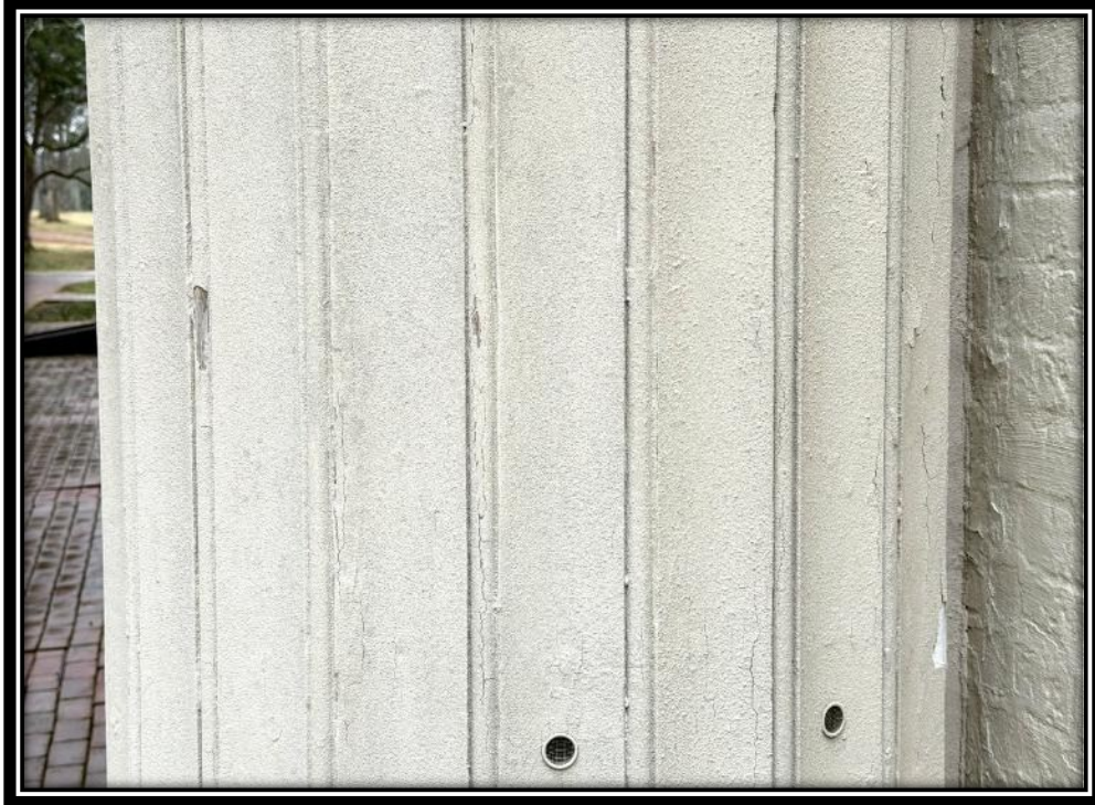
The sand painted finish on the front columns of the Hermitage mansion is cracking and paint is beginning to fail in areas, December 2025.
