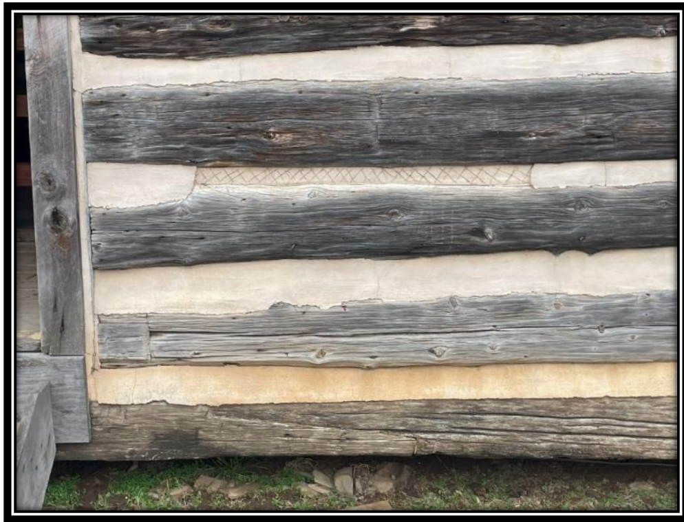
Typical daubing deterioration at Alfred's Cabin, December 2024.
