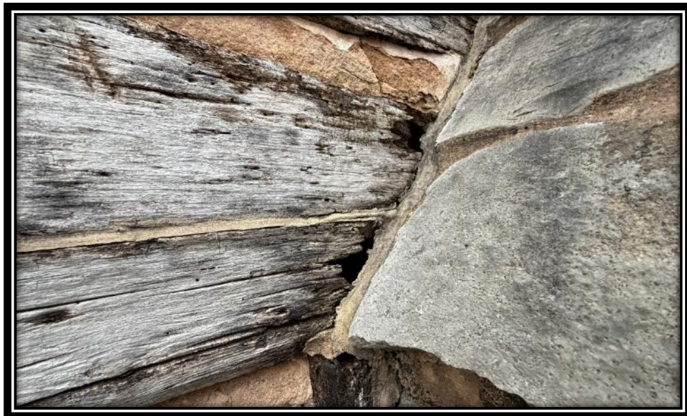
North elevation of Kitchen showing deteriorated log end at Kitchen chimney that requires patching, December 2025.
