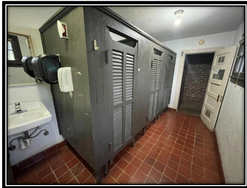
Antiquated non-accessible Maintenance Building women's public restroom, October 2025.
