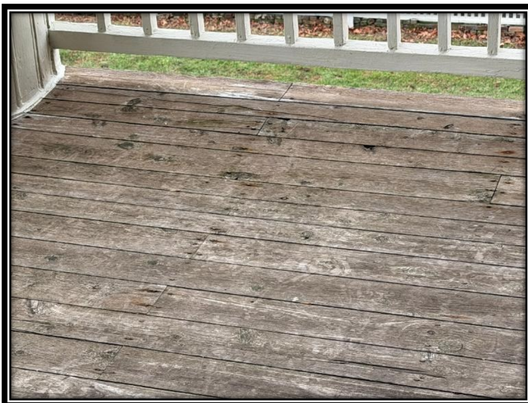
The Hermitage mansion has two second-floor porches with deteriorating floorboards. The beam and joist support structure under the floors should also be inspected.
