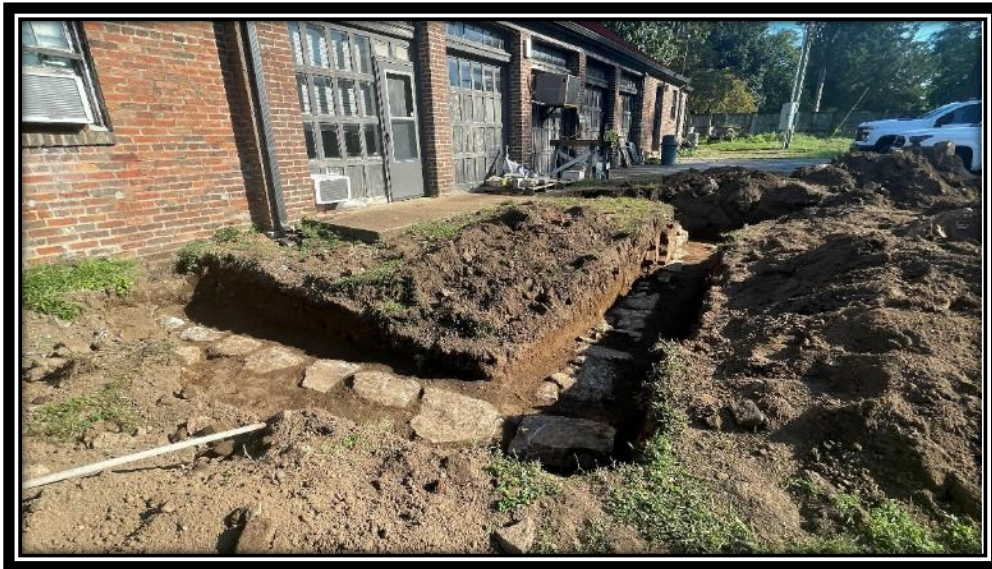
Exposed foundation of Jackson's brick Carriage House and Stable proves it continues under the Maintenance Building, October 2024.
