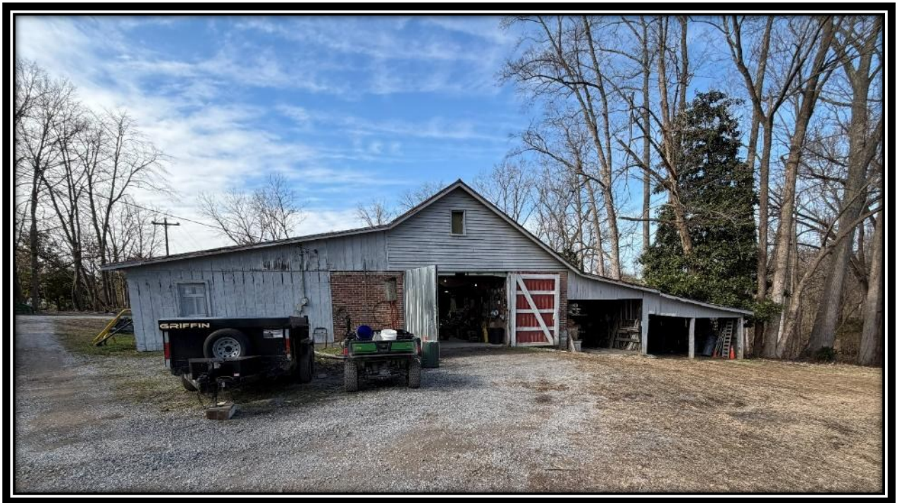
East elevation of the Storage Barn, showing storage room on south side and open bay storage on north side that will be demolished, December 2025.
