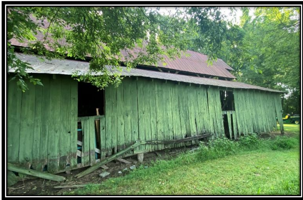
East Field Barn, west elevation, note that the wall is lifted up due to the building's lean to the east, September 2025.
