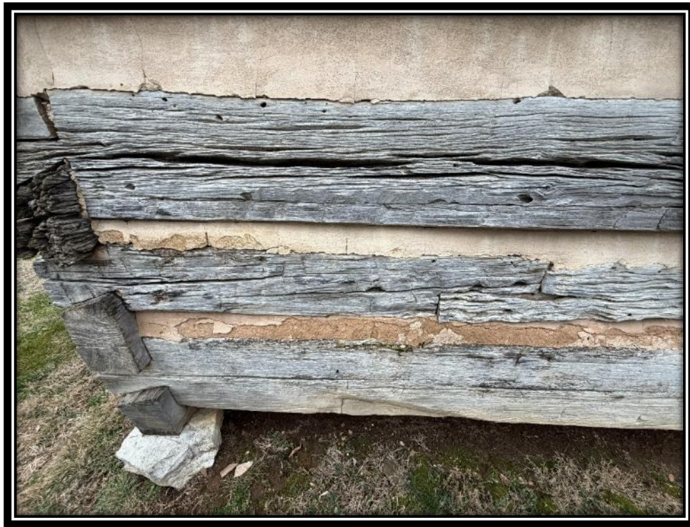
Deteriorated daubing on the north elevation of the First Hermitage Farmhouse, December 2025.
