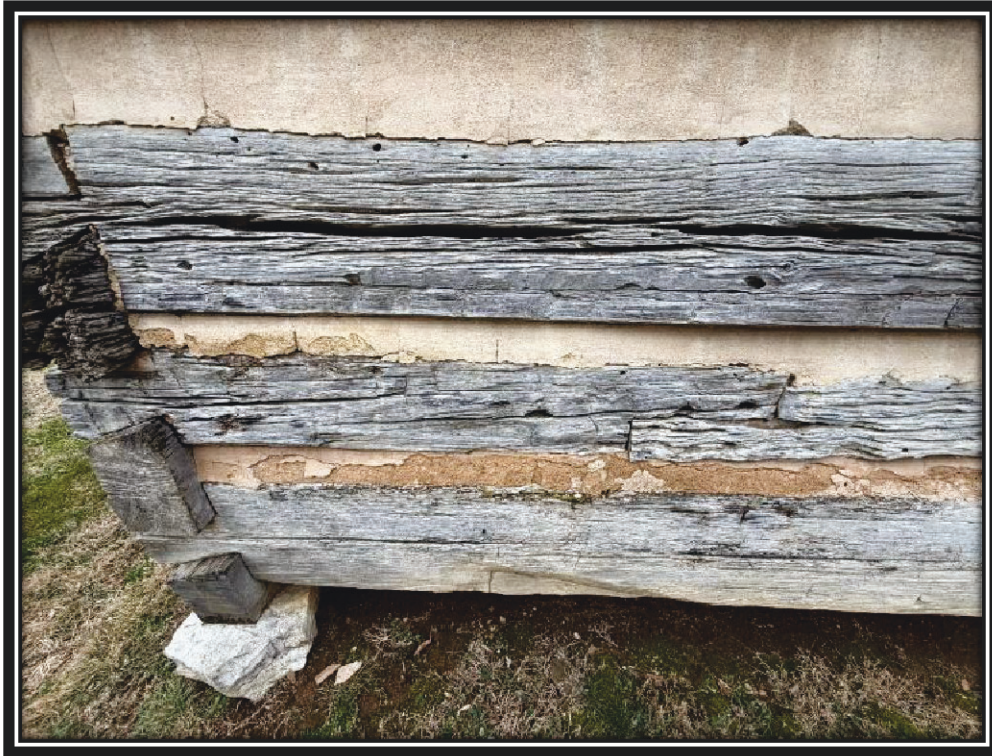
Deteriorated daubing on the north elevation of the First Hermitage Farmhouse, December 2025.
