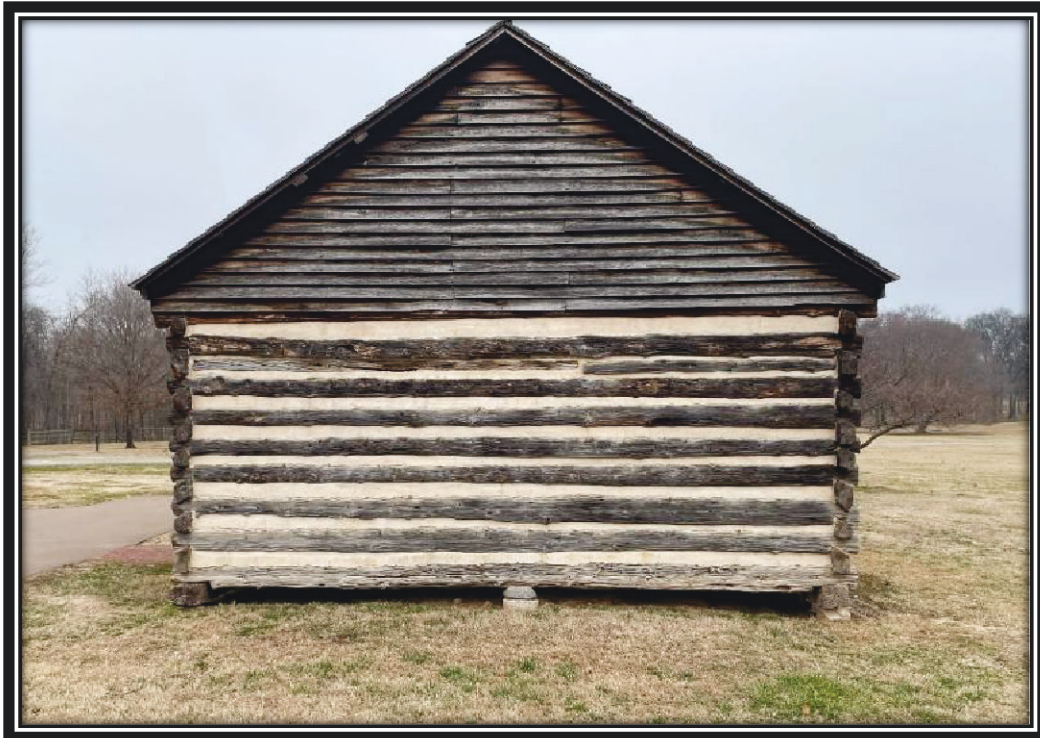
Deteriorated gable siding pulling free from wallowed out nail holes, December 2024.
