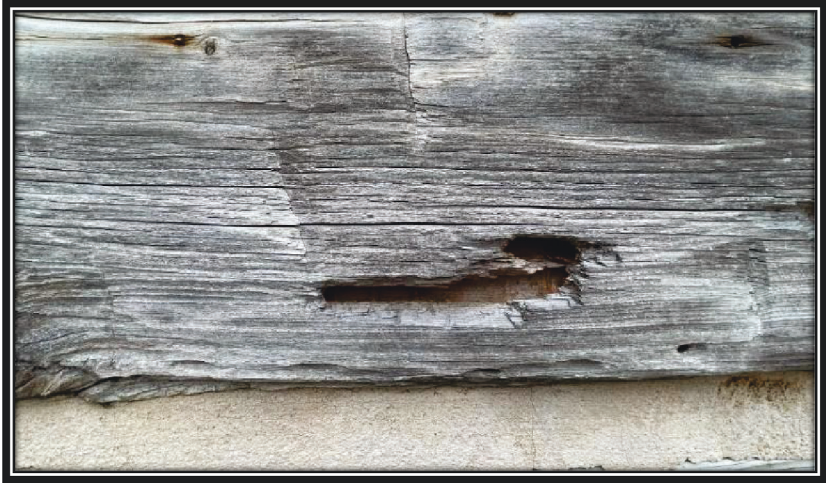
Before, typical log damage at Alfred's Cabin that requires patching to keep water from pooling inside the log cavity, December 2024.
