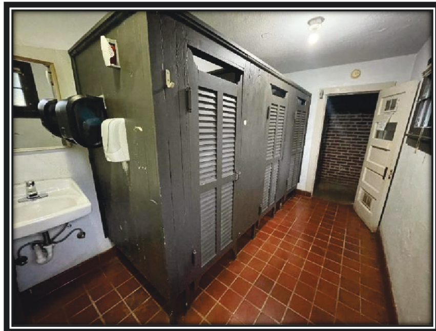
Antiquated non-accessible Maintenance Building women's public restroom, October 2025.
