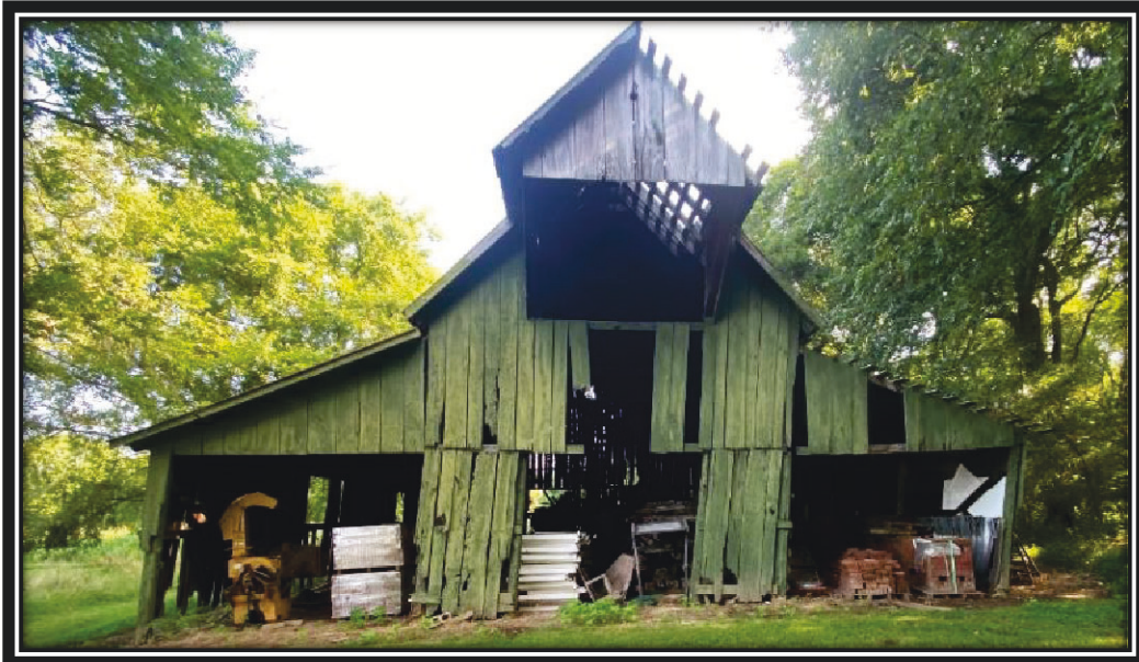
East Field Barn condition September 2025. Note lean of building to the east and missing metal roof panels and wood siding, September 2025.
