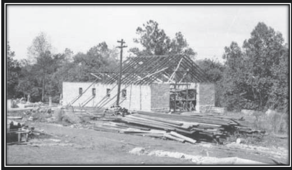
Brick Storage Barn under construction in 1936. This original brick portion of the barn will be retained.
