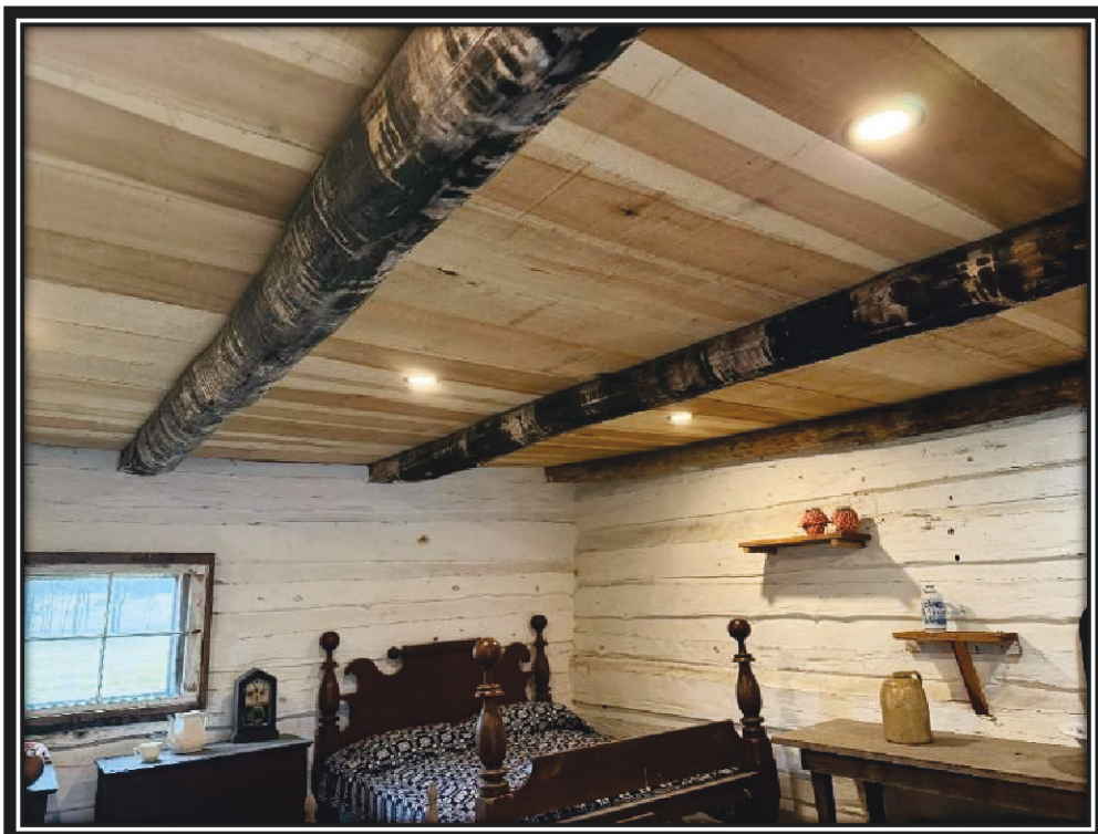
The non-original bead board ceiling in Alfred's Cabin was replaced with a historically appropriate Tulip Poplar wood plank ceiling, December 2025.
