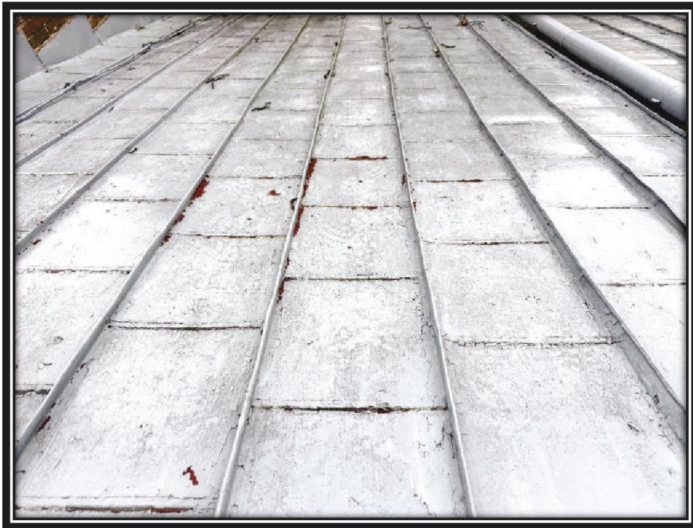
Roof paint on the Hermitage's west wing roof shows cracking and chipping, December 2025.
