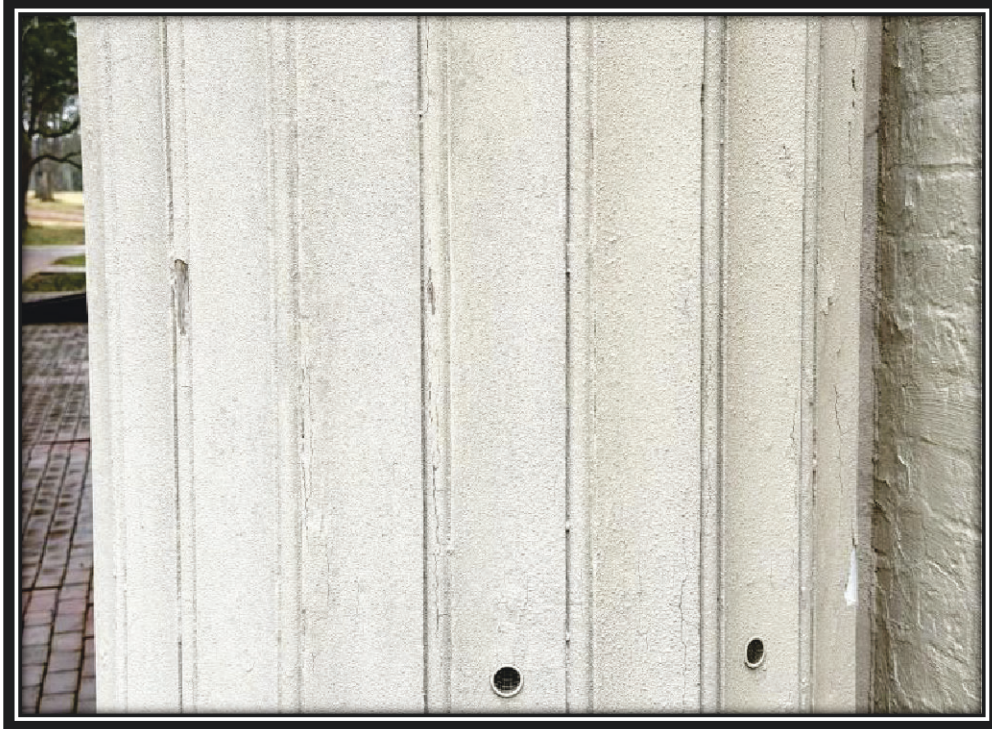
The sand painted finish on the front columns of the Hermitage mansion is cracking and paint is beginning to fail in areas, December 2025.
