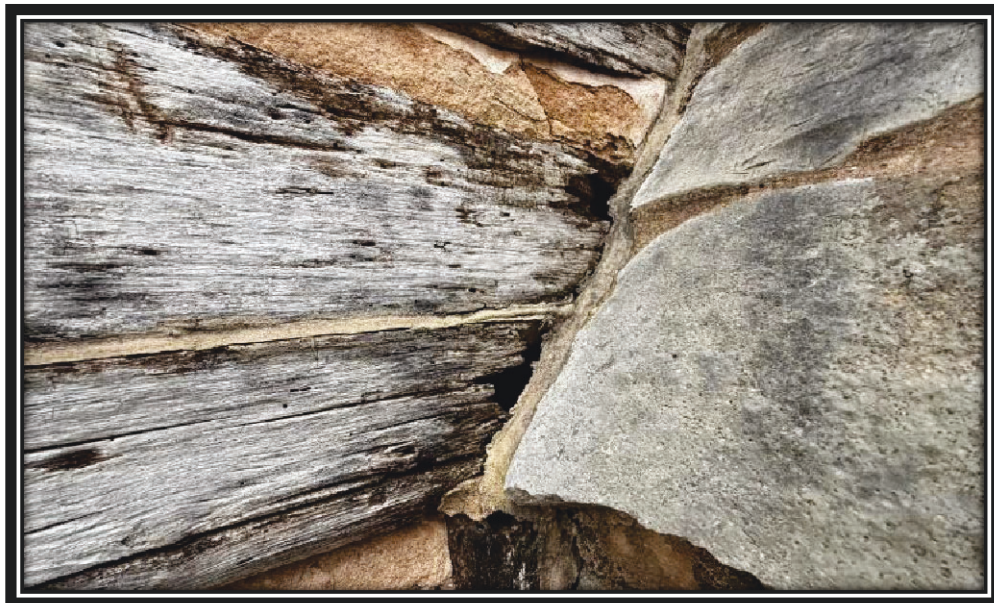
North elevation of Kitchen showing deteriorated log end at Kitchen chimney that requires patching, December 2025.
