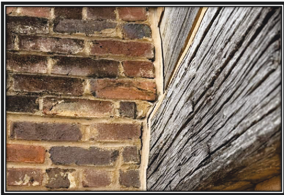
Failed elastomeric sealant expansion joint between the log walls and brick chimney of the First Hermitage Farmhouse, December 2025.
