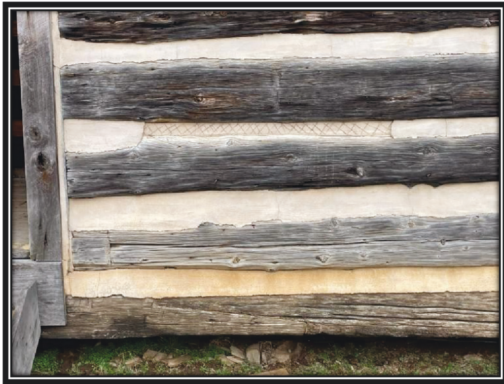
Typical daubing deterioration at Alfred's Cabin, December 2024.
