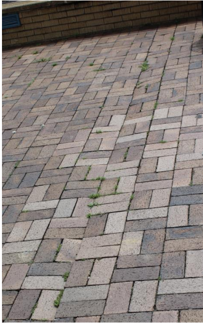
Photograph 7 – Brick paver deterioration
