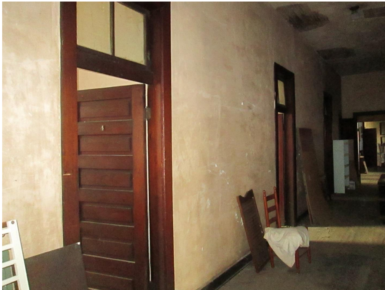
Photograph 19. First floor hallway in the Kefauver Hotel, showing room entries with transoms, facing southeast.
