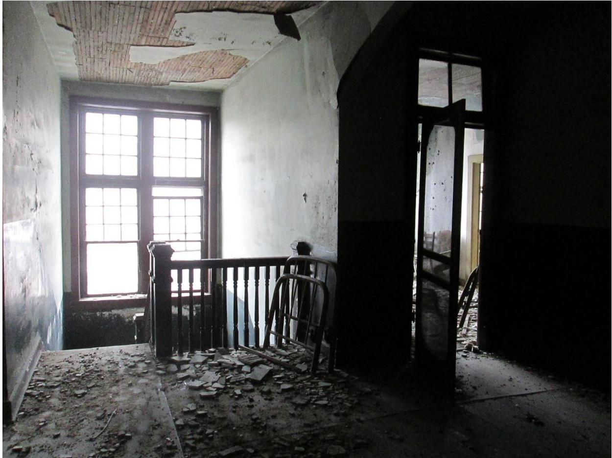
Photograph 26. Front stairway, landing, and office space (at right) on the second floor of the Kefauver Hotel, facing south-southwest.
