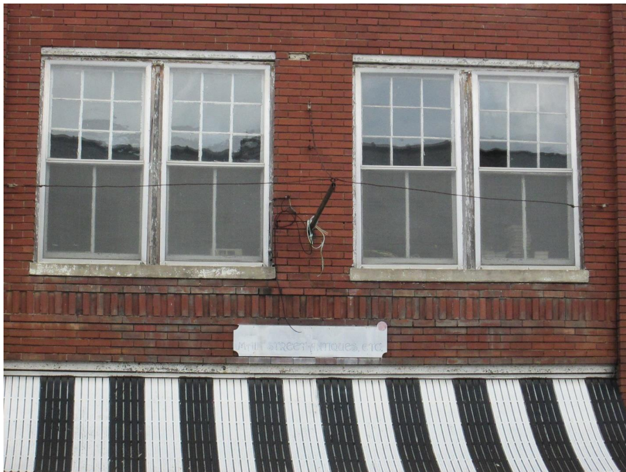
Photograph 8. Detail of windows on façade (south elevation) on the Kefauver Hotel, facing north.
