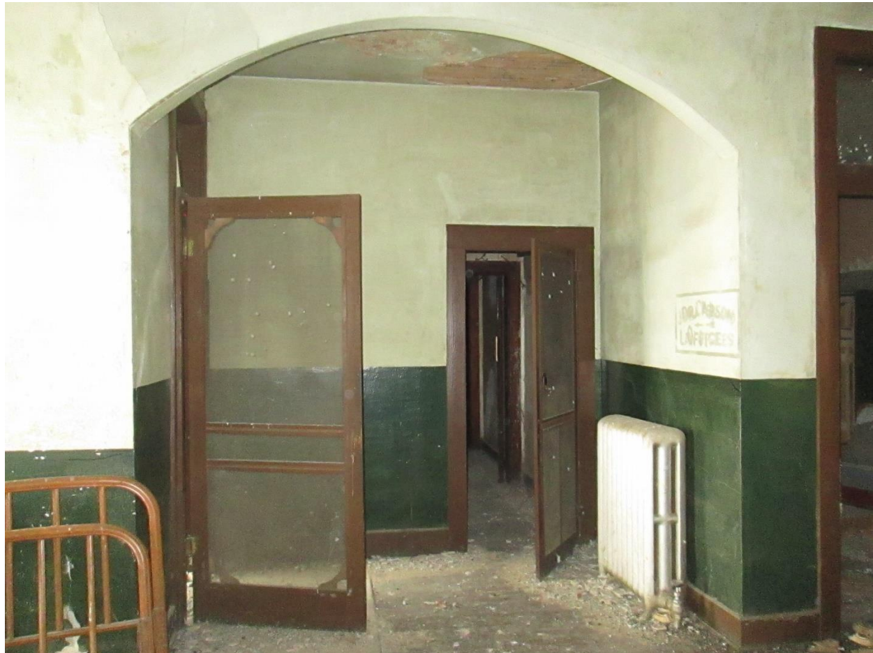
Photograph 24. Office spaces located on the second floor of Kefauver Hotel, facing west.
