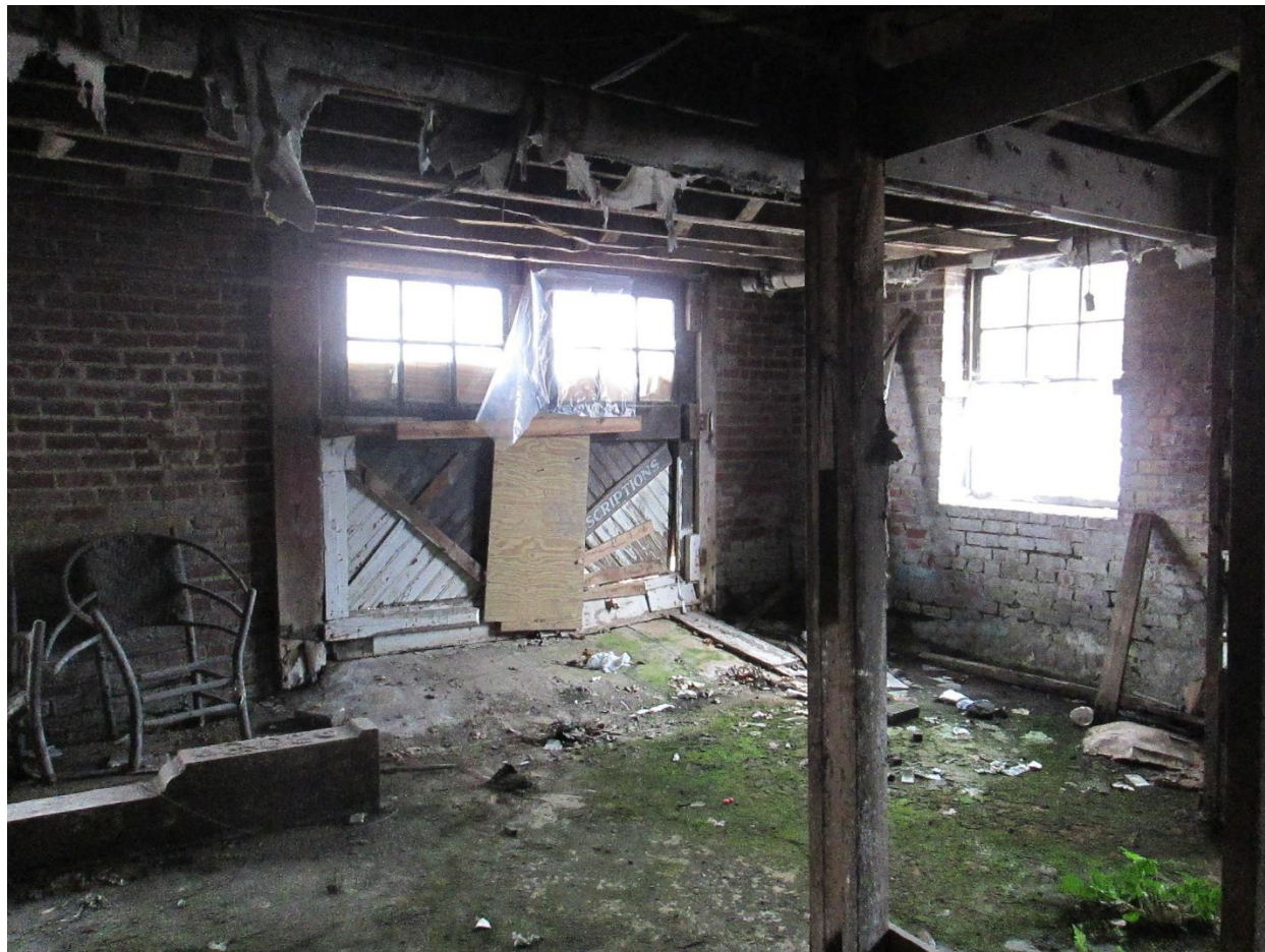
Photograph 30. Portion of unfinished basement in the Kefauver Hotel, showing original double-leaf vehicular entry, facing northeast.
