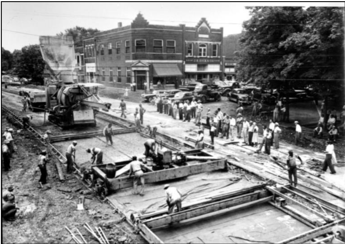
Figure 3: Paving of the Memphis to Bristol Highway (Tennessee State Route 1) in Sparta, Tennessee, ca. 1949. Courtesy of the Tennessee State Library and Archives.
