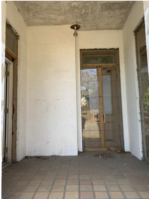
Photo 2, Front façade, Inset Entryway. Three single leaf doorways. Only central door is original, all have original transoms
