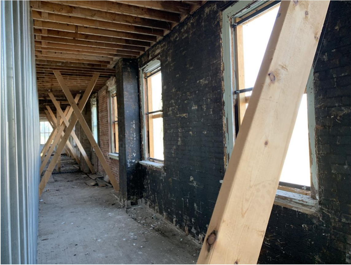
Photo 17, first floor, east wall front rear of building. Opposite wall has same conditions
