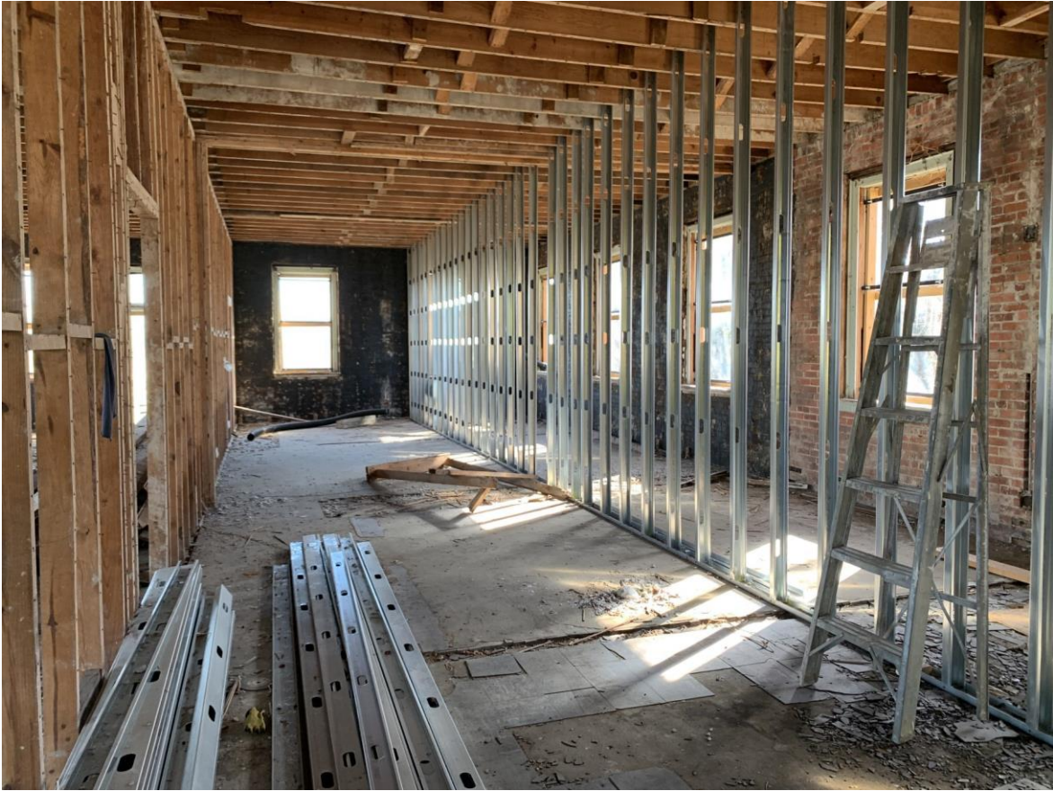
Photo 21, second floor, facing rear and east walls from front of building (stairs to left). Wood flooring and tile finishes remain in portions
