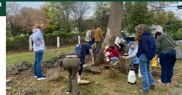
Hands on repairs by attendees at cemetery conservator Terry Minton's recent workshop in Old Hickory at the Thomas Overton Cemetery.
