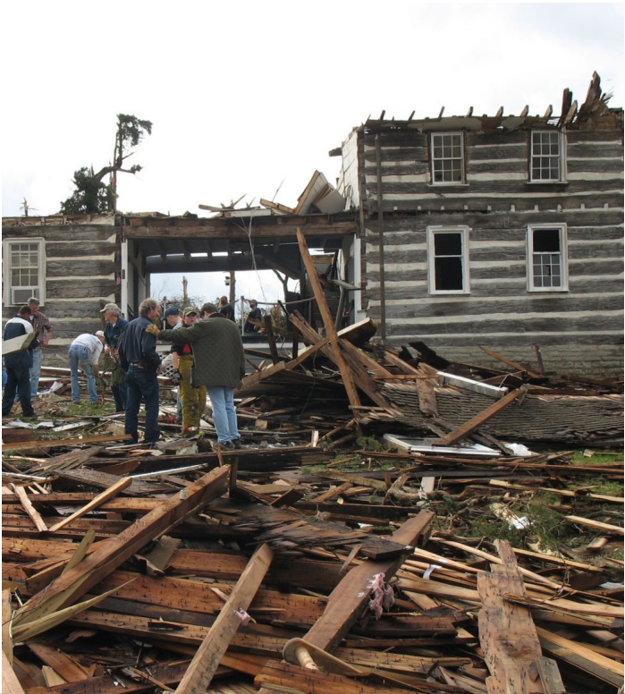
Patrick McIntyre at Wynnewood State Historic Site assessing tornado damage on the morning of February 6, 2008.
