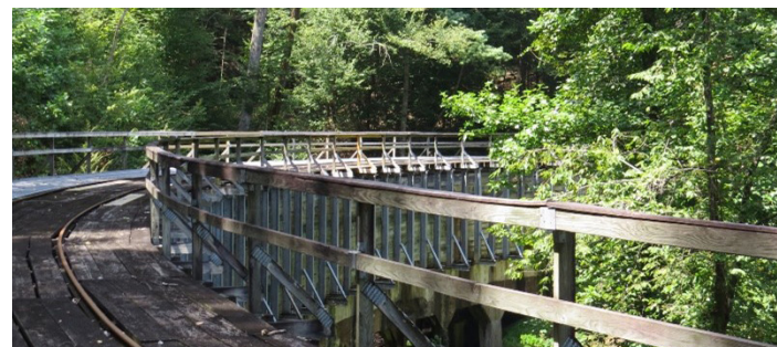
Section of the Ocoee No. 2 wooden flume, 2023. Photo courtesy of Caty Dirksen.
