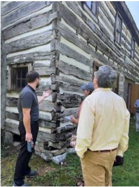
Executive Director McIntyre and Mr. Cooley Inspect Building Conditions at the ca. 1803 Historic Browns Ferry Tavern in Chattanooga.
