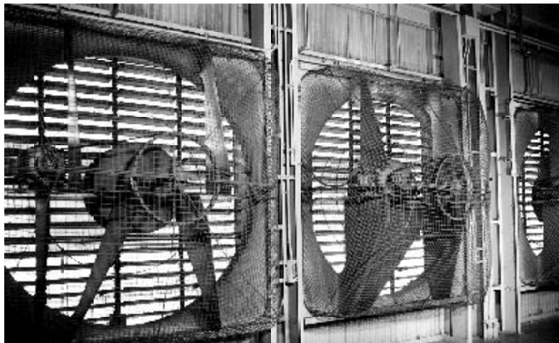
Six-foot diameter fans were installed in Colex Building 9201-5 in 1956 to increase ventilation and reduce worker exposures.
