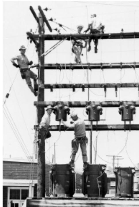
Because much electricity was used at the ORR, components containing PCBs were plentiful.
