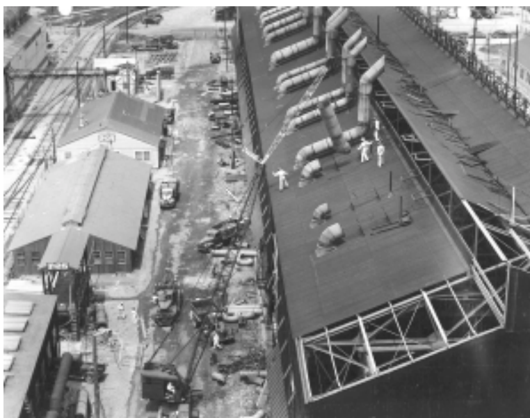
Workers disassemble the main process building of the S-50 Plant in the 1940s. The S-50 liquid thermal diffusion process for enrichment of uranium was abandoned after about one year.
