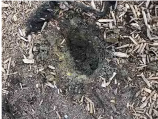
Photo 3: High traffic area, beneath the swing set located within the playground area in the northwest corner, where a soil/mulch mix was observed and the geotextile fabric was compromised (CLX-SL-PGIN-13)
