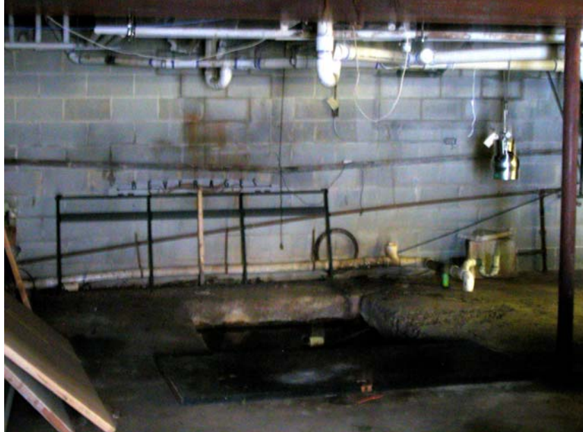
FIGURE 2 - Photo of the sump in the basement, Concord Cleaners, 3706 Hillsboro Pike. Nashville, Davidson County, Tennessee. (Photo credit: David Borowski, TDH, 1/19/05)
