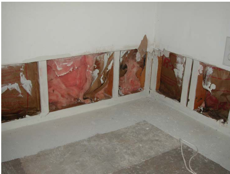
Figure 2. View of the drywall removal from the bottom 12 inches of the walls.
