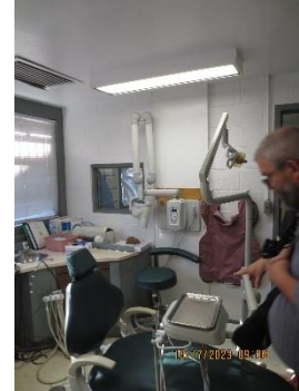
E2 – Infirmery Typical Lighting
