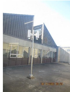
E4 – Courtyard Pole Lighting
