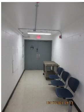
E5 – Surface Mounted Wiring
