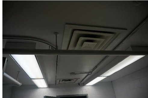
M2 – Supply Diffuser
