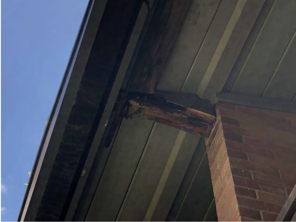
Photograph 5 – Decay at wood beam at lodge roof eave.
