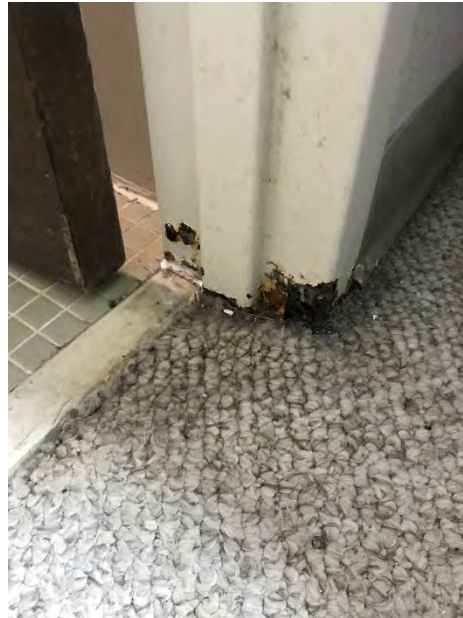
85) Guest Room 107 – Resting of bathroom door jamb at base.
