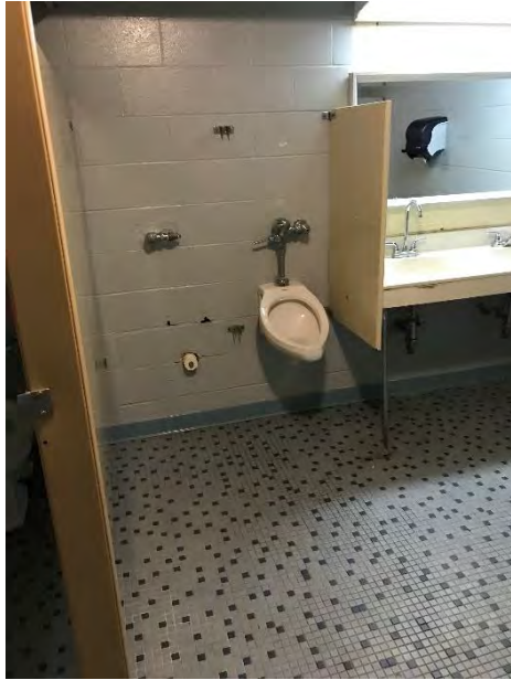
67) First Floor Men's Room – Restroom is dated and does not meet ADA requirements
