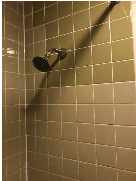
87) Guest Room 107 – Miss-matched tile color from previous repairs.
