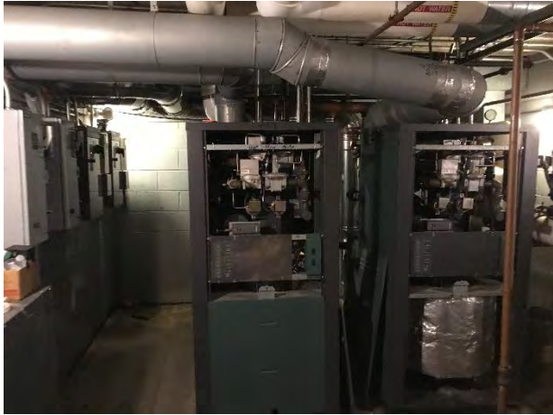
184) Second Floor Mechanical Room
