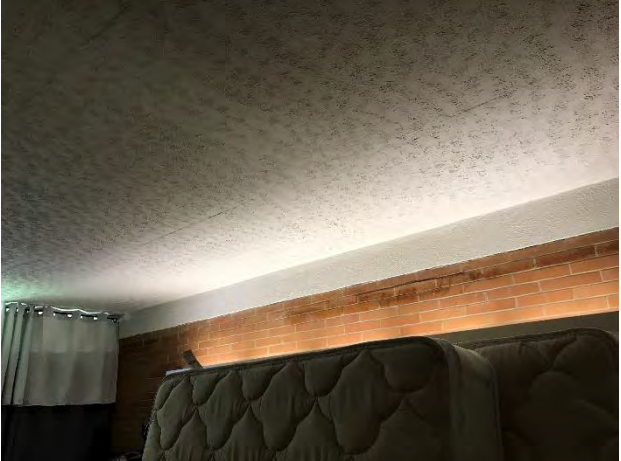
81) Guest Room 107 – View of headboard lighting.
