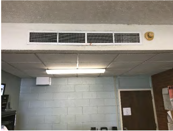
41) Lobby Office - Air distribution grille.
