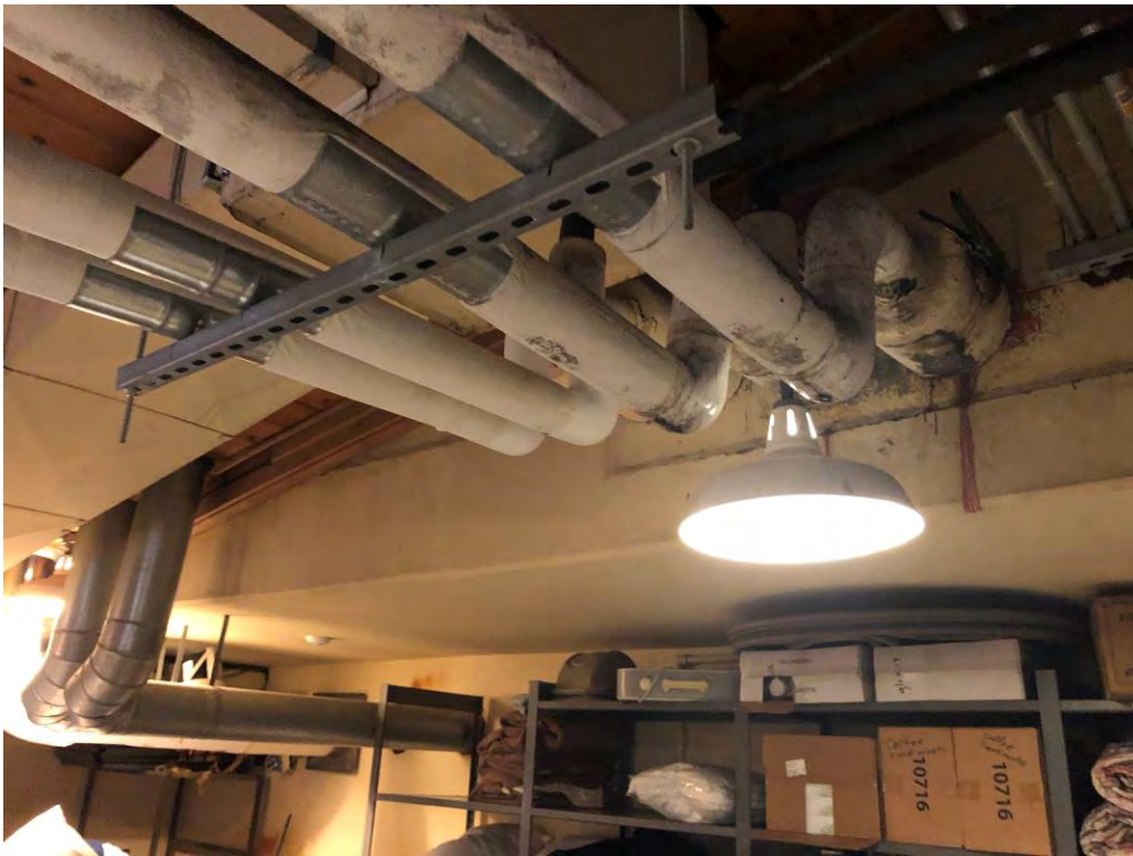
Photograph 12 – Concrete slab supporting mechanical equipment above second floor mechanical room at lodge.
