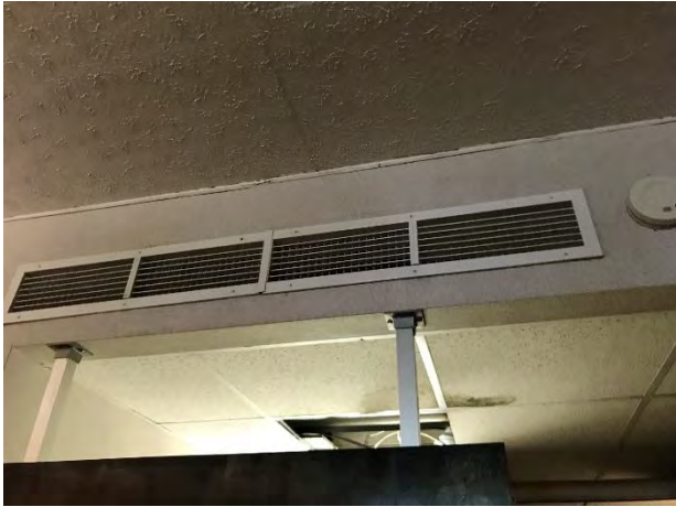
82) Guest Room 107 – View of air distribution grille.
