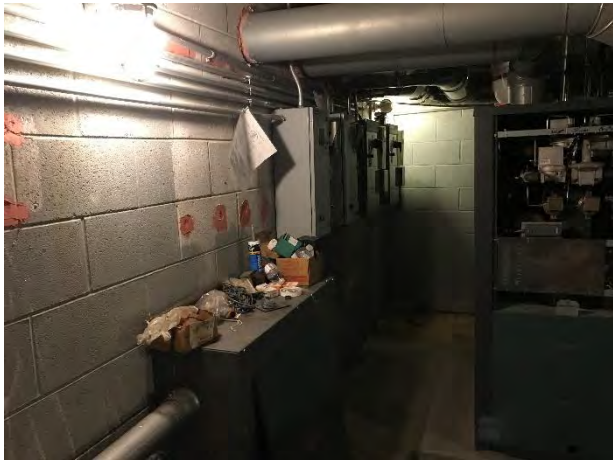
186) Second Floor Mechanical Room
