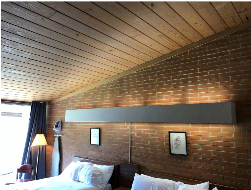
Photograph 10 – Typical second floor room at lodge. Wood roof decking and load bearing masonry walls
