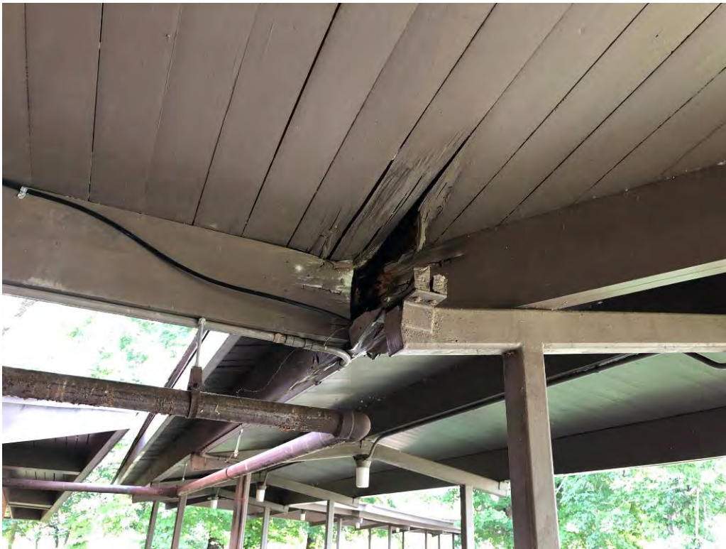
Photograph 18 – Wood decay at covered walkway between lodge and motel.
