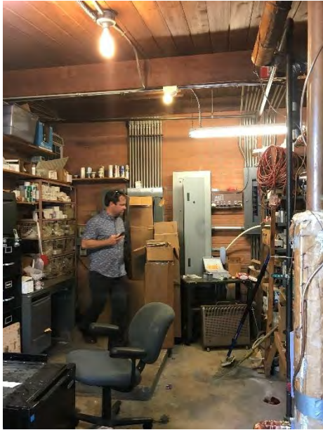
217) Motor Court Mechanical Room
