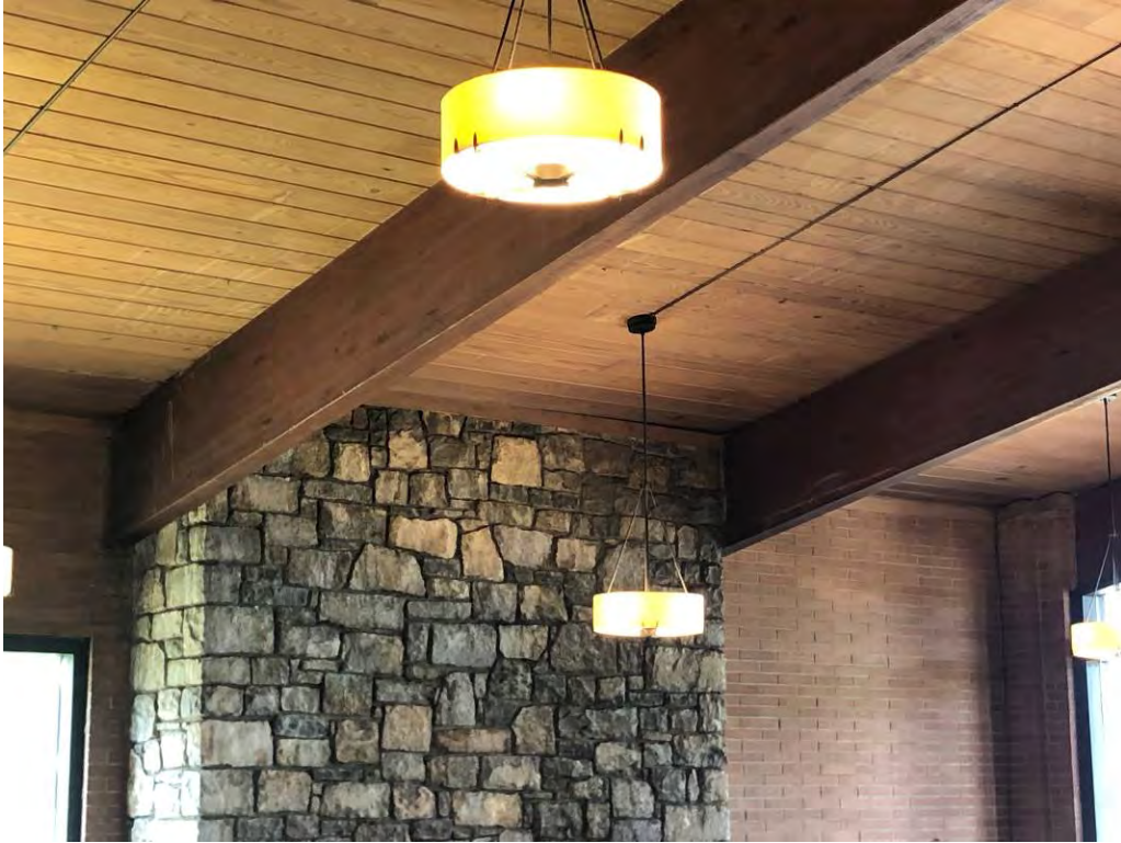
Photograph 7 – Roof framing at fireplace in lodge lobby. Potential water damage at roof decking and wood beams.
