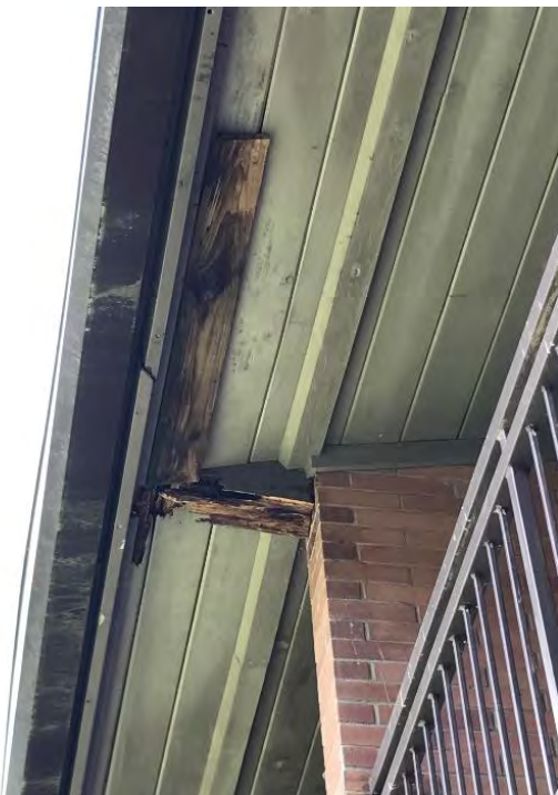
19) Lodge Exterior – View of rotting wood at the north facing façade.
