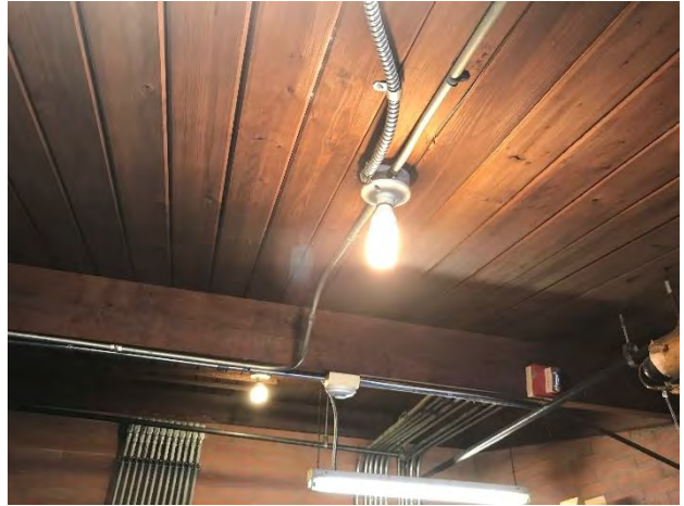
222) Motor Court Mechanical Room
