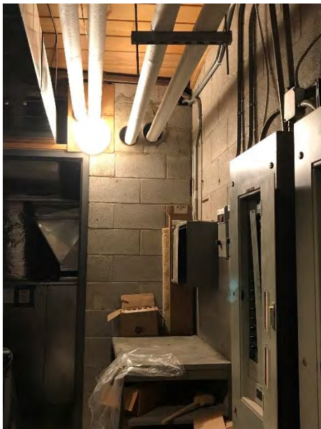
178) Second Floor Janitor / Electrical
