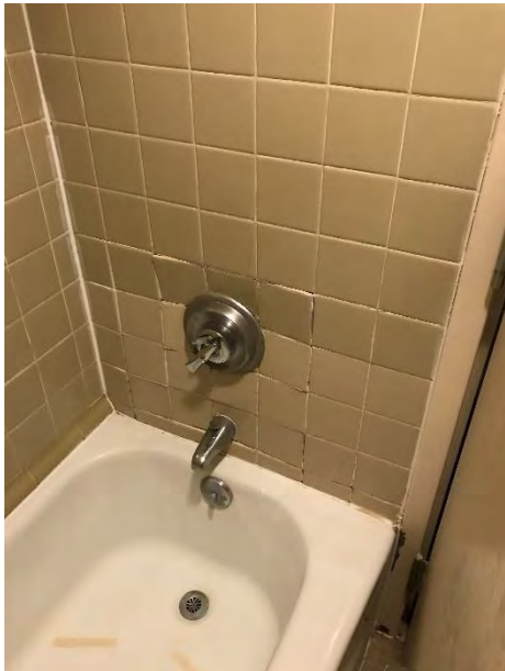
86) Guest Room 107 – View of deteriorating wall substrate at control valve.
