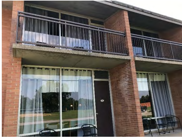
17) Lodge Exterior – View of guestrooms facing east. Note masonry staining and efflorescence.
