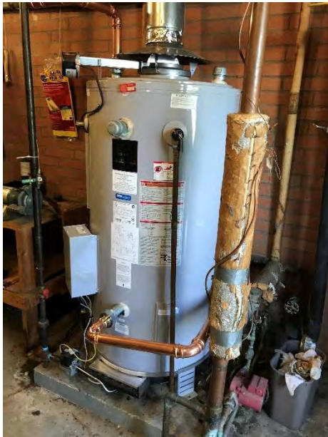
219) Motor Court Mechanical Room
