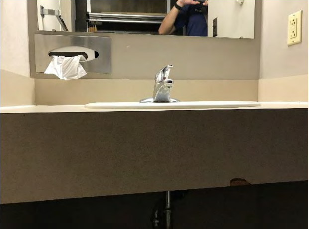
83) Guest Room 107 – Sink counter – Note plumbing pipes below are not wrapped.
