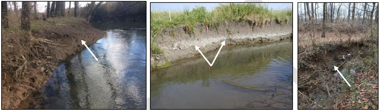
Figure 6.22. Photos showing fluvial erosion on streambanks.
