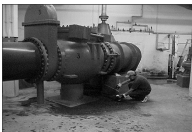
Return Activated Sludge Systems
