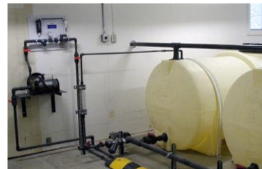
Chemical Storage and Feeders
