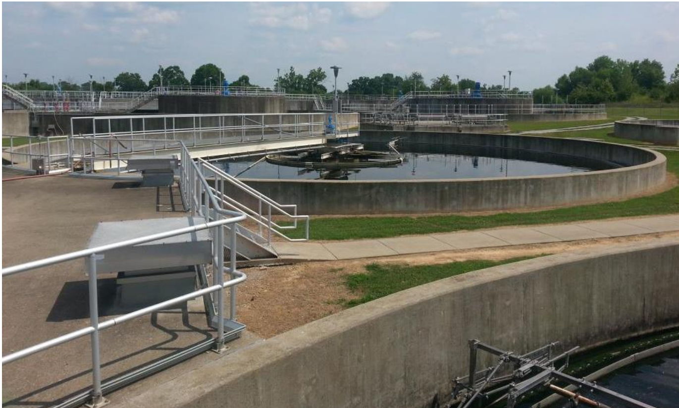
City of Franklin Wastewater Treatment Plant
