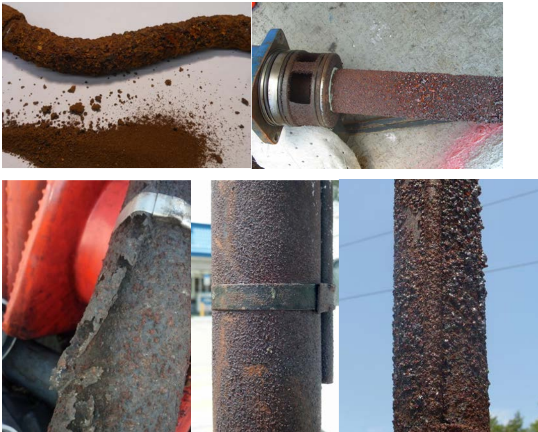
Figure 9: Microbially influenced corrosion of fuel storage and dispensing systems (Sources in clockwise order: Marathon Petroleum, Fuel Quality Services, Fuel Quality Services, Fuel Quality Services, Steel Tank Institute)
