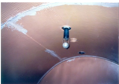
Flow Restriction (Ball Float Valve)*
