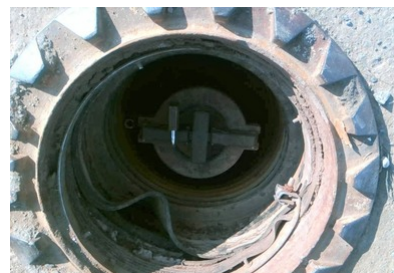
Deformed spill bucket wall
