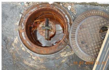
Corroded spill bucket full of liquid
