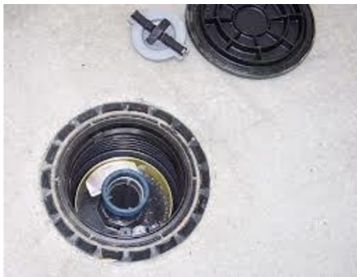
Properly maintained spill bucket
