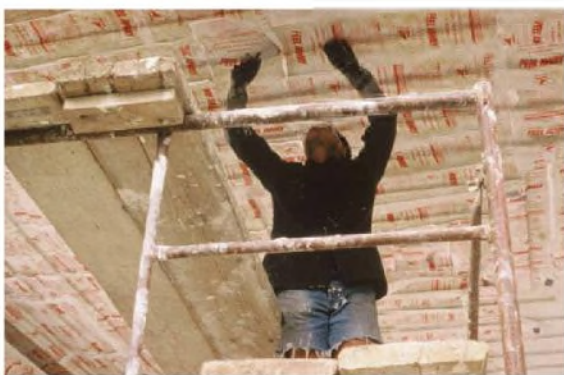
FIGURE 8.6 Inadequate worker protection during a large overhead paint stripping project. Depending on exposure, this worker should be wearing protective clothing, long chemical-resistant gloves and a respirator; and should also be protected against falls.
