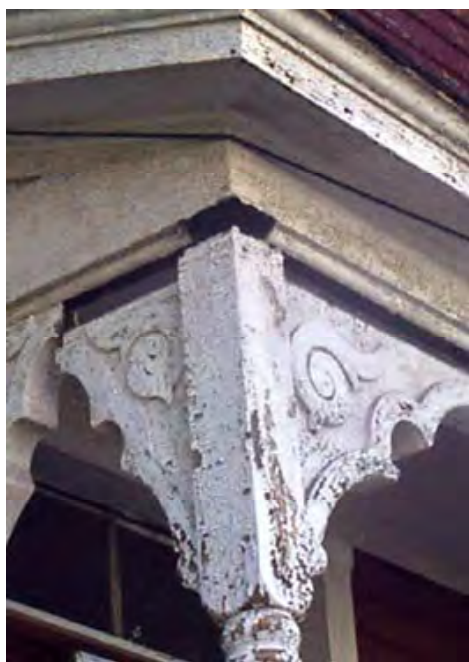
FIGURE 1.2 Deteriorated residential paint on house trim.
