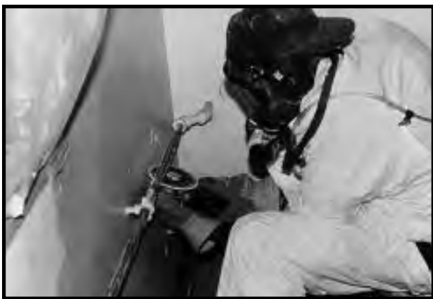
Figure 12.12b Open-Faced Power Sanding or Grinding Is Prohibited.
