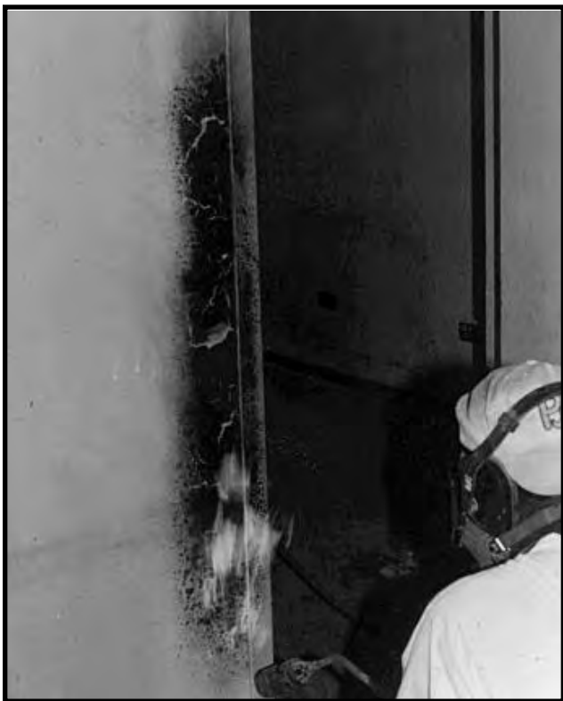
Figure 12.12a Open Flame Burning Is Prohibited.
