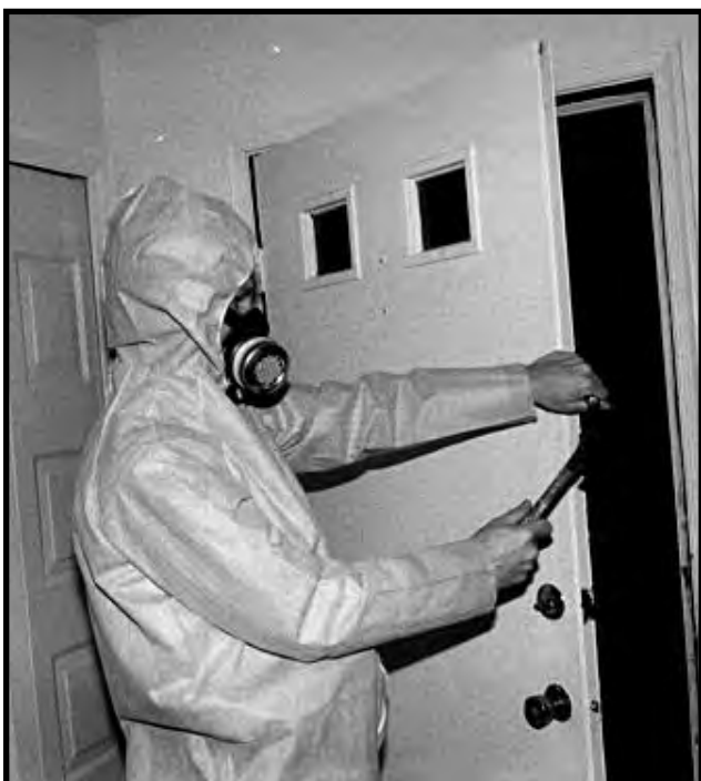
Figure 12.21 Use Punches To Identify the Location of Components Before Sending Them Offsite for Paint Removal.
