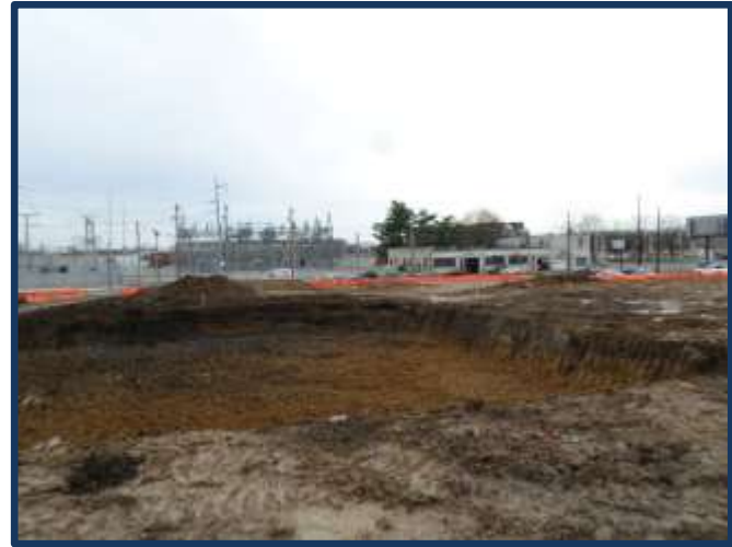
This photograph shows the initial excavation under the former Laycook Clutch building after the slab was removed.
