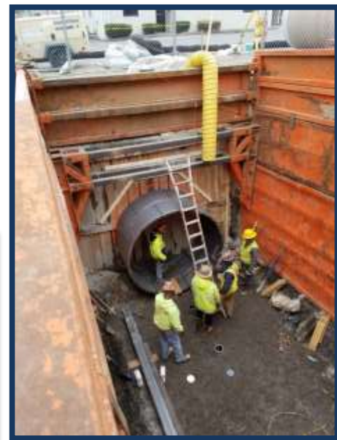
Above is the tunnel portion of the alignment, preparing to begin excavation.
