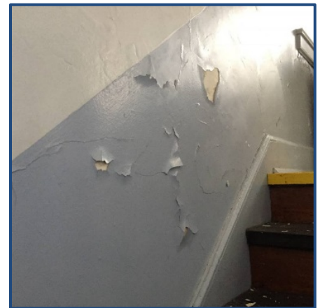
Lead-based paint was found throughout the building prior to being addressed.
